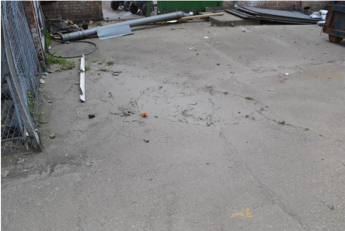
Silt in location of previous ponding on the site
