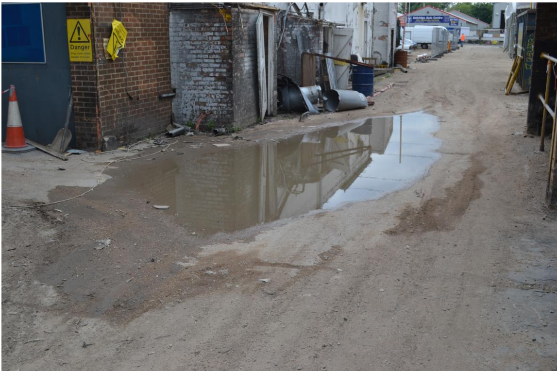
Surface water ponding on site at location of surveyed soakaway
