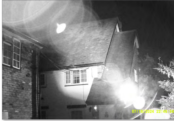
Photograph of northern and eastern elevations of Building 3 at end of survey 4
