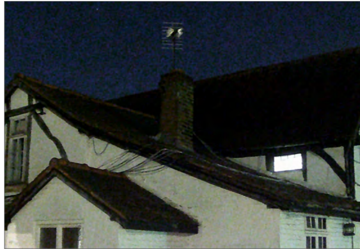
Photograph of southern and eastern elevations of Building 2 at end of survey 1
