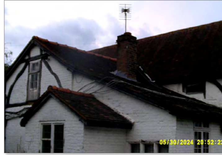
Photograph of southern and eastern elevations of Building 2 at start of survey 2
