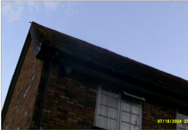
Photograph of northern and eastern elevations of Building 4 at start of survey 4
