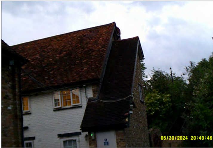
Photograph of northern and eastern elevations of Building 3 at start of survey 2
