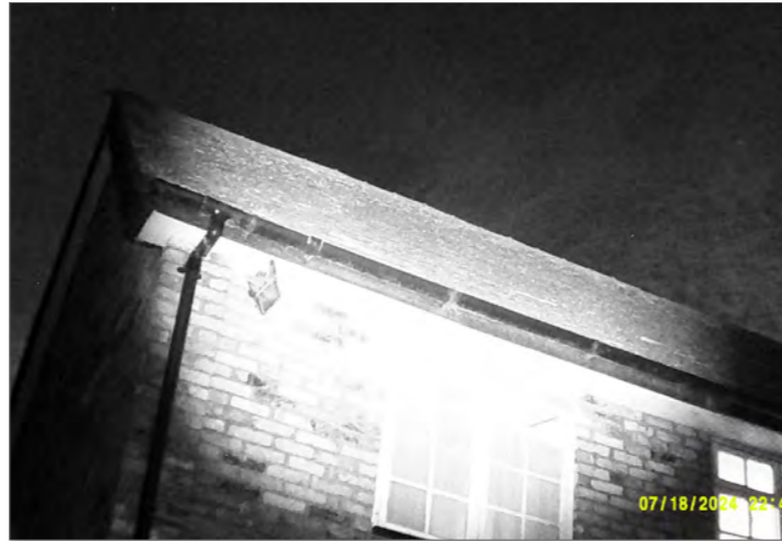
Photograph of northern and eastern elevations of Building 4 at end of survey 4
