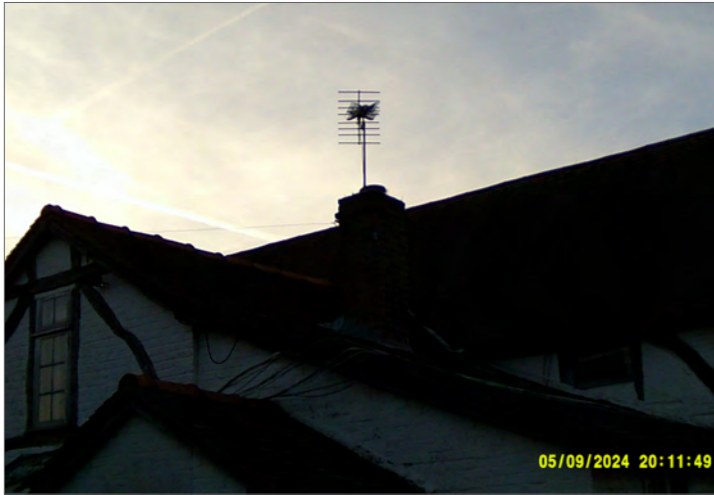
Photograph of southern and eastern elevations of Building 2 at start of survey 1
