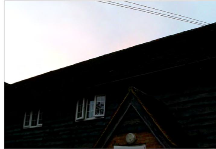
Photograph of eastern section of the southern elevation of Building 3 at start of survey 2
