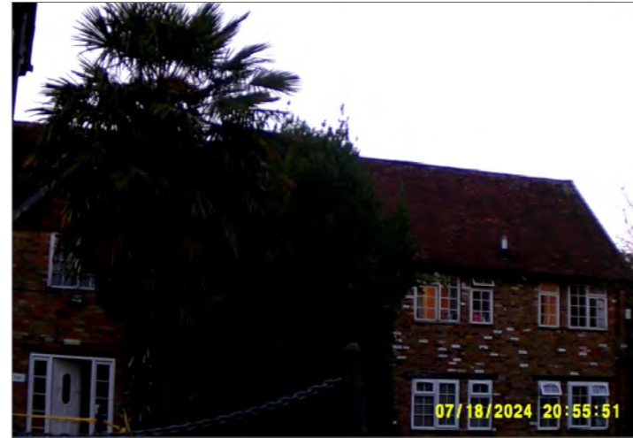
Photograph of eastern sections of the southern elevation of Building 4 at start of survey 4
