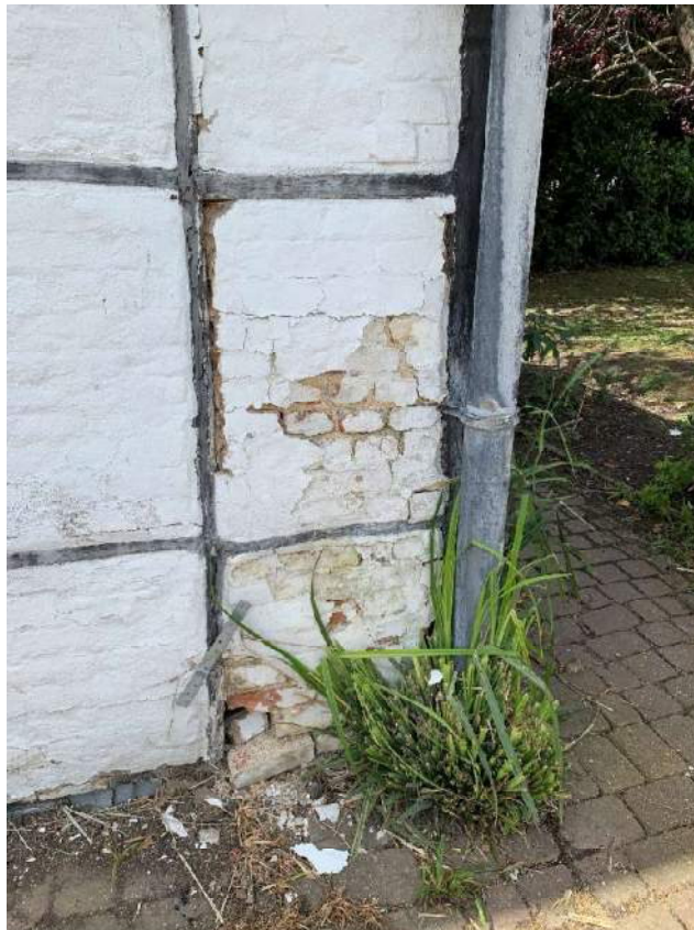
Photograph 4 – Friable masonry to north eastern corner
