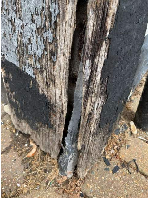
Photograph 11 – Decayed base to corner cladding
