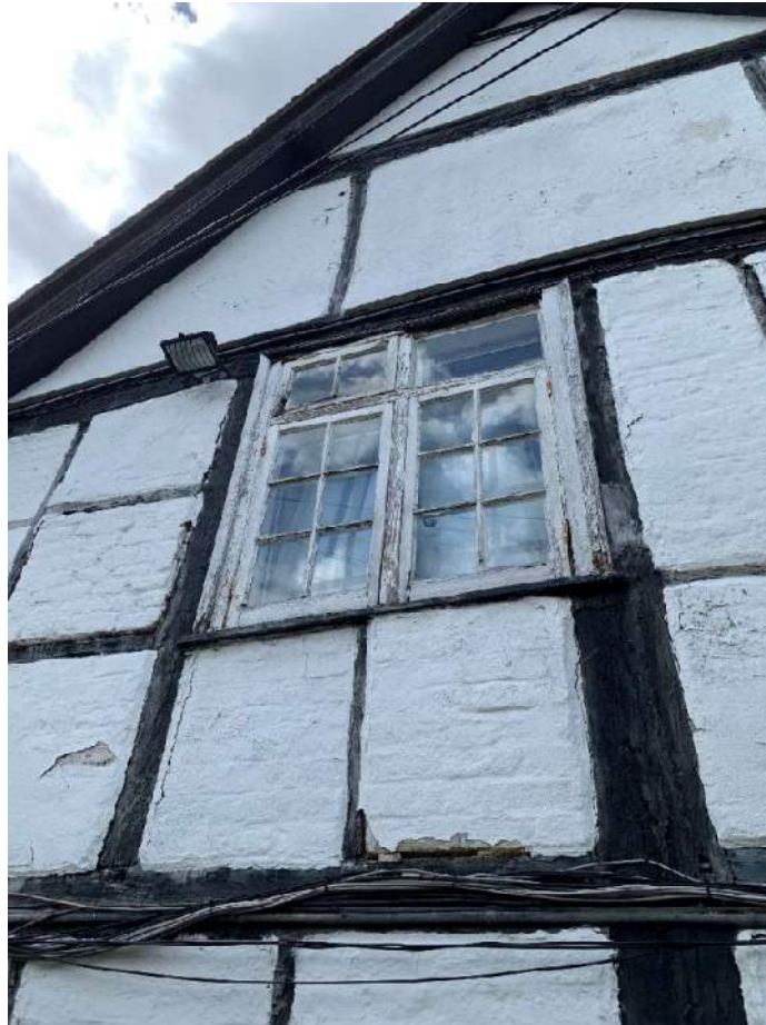
Photograph 5 – decayed window frame
