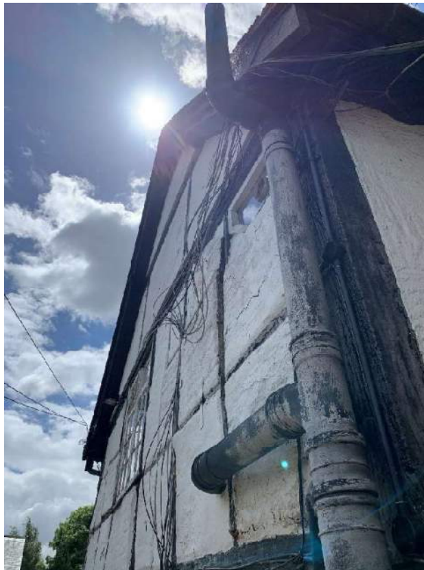
Photograph 3 – Showing distortion to upper panels
