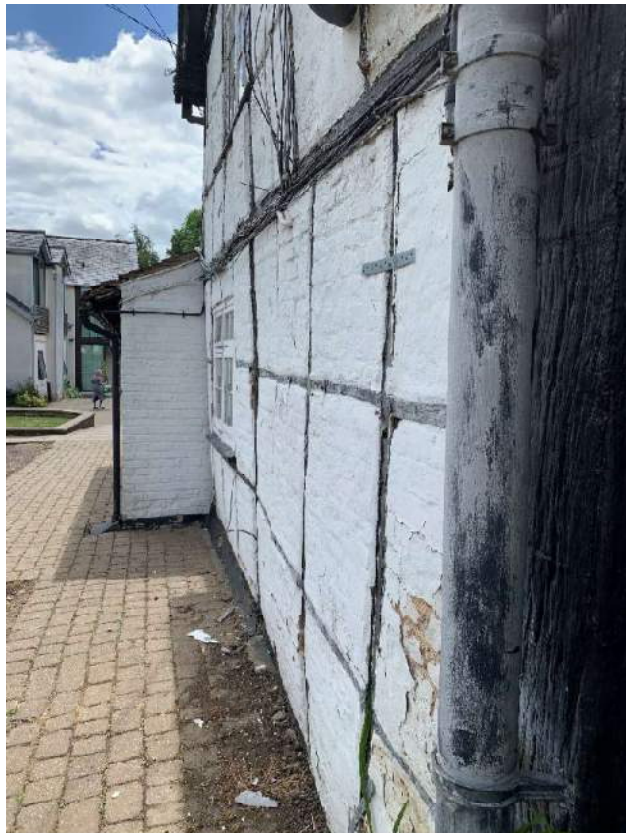
Photograph 2 – Showing distortion to lower panels
