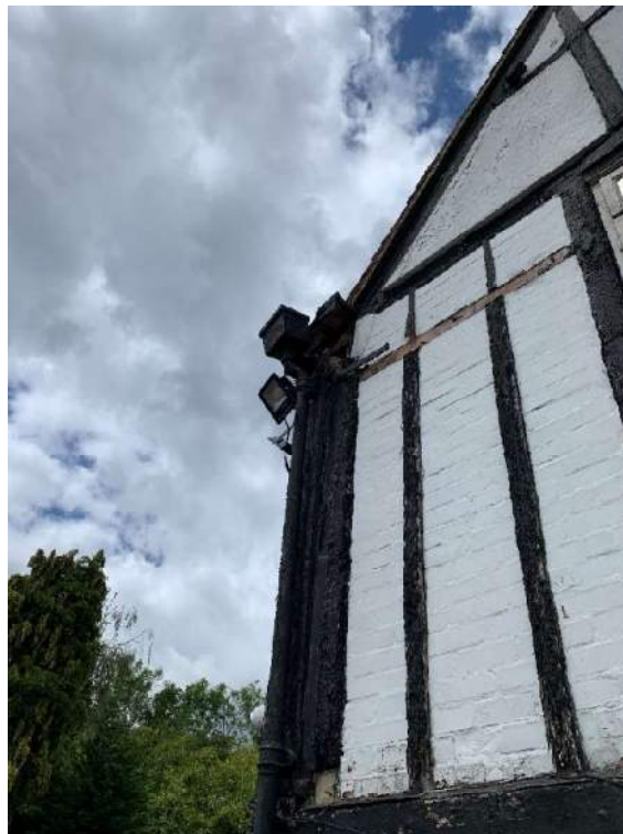
Photograph 10 – Dislodged cladding and hopper
