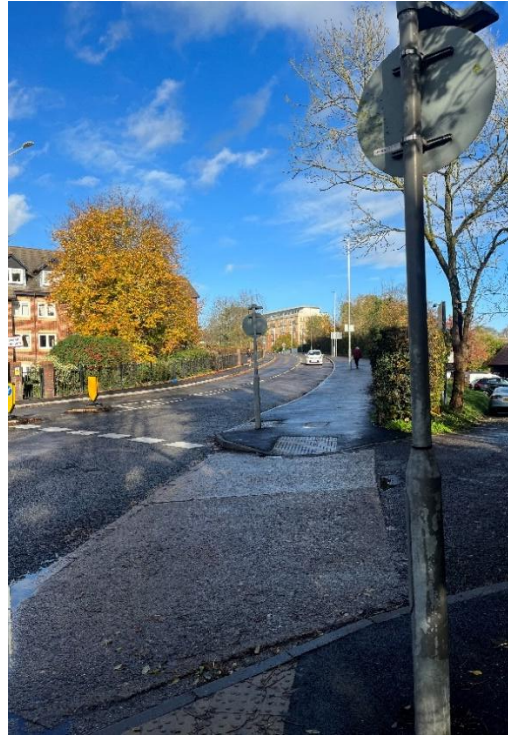
Photograph 4: Existing footway conditions on West End Road
