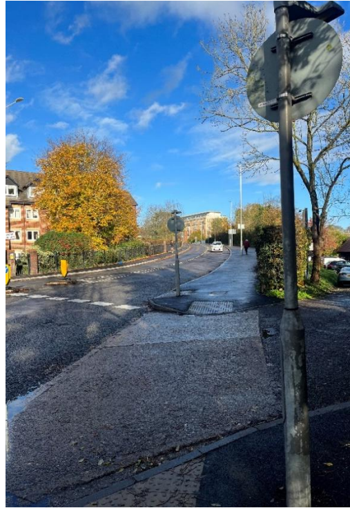
Photograph 4: Existing footway conditions on West End Road
