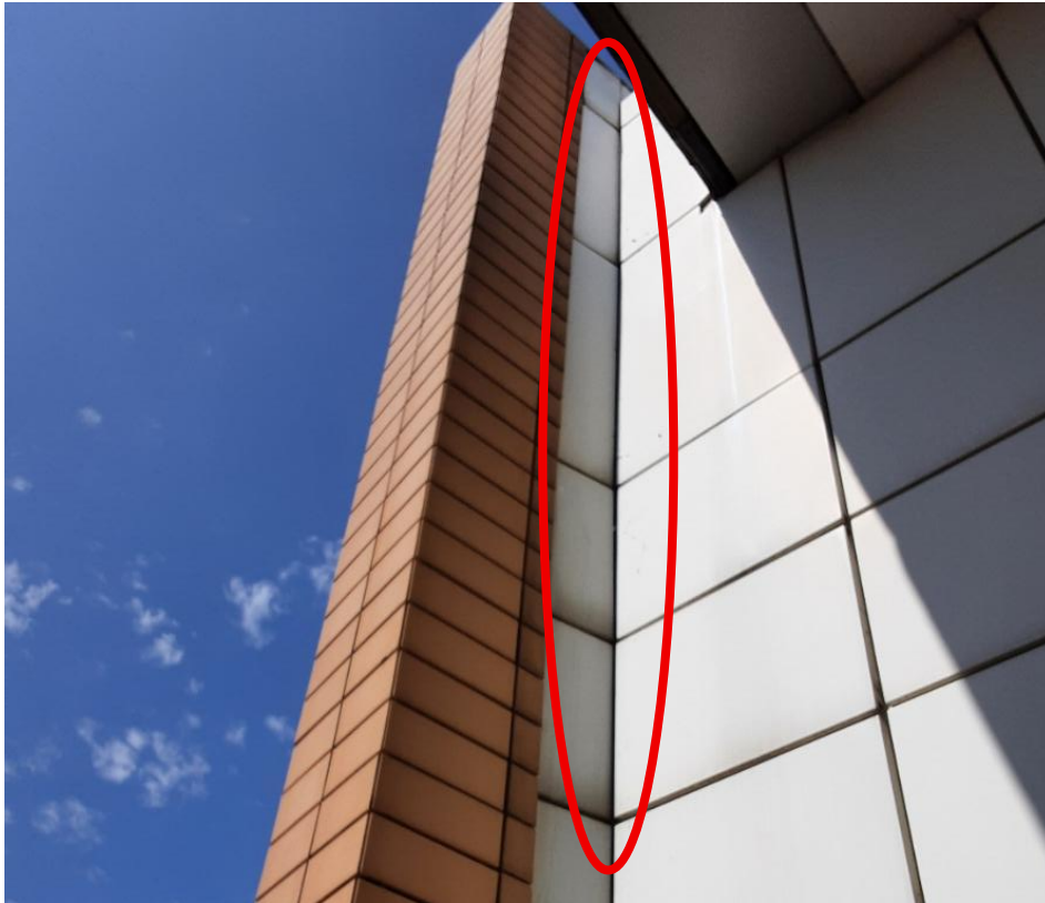
Photograph 9: PRF2 – Gaps leading to suitable sized space behind cladding (western aspect of B2)
