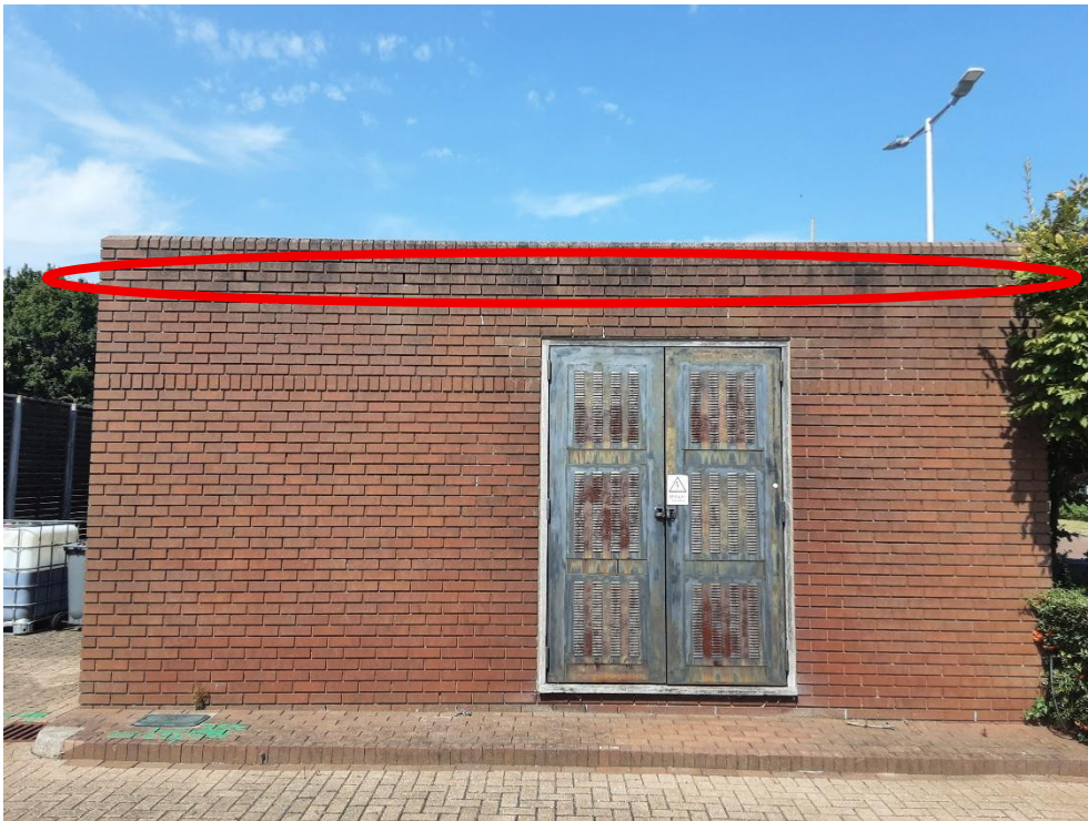
Photograph 12: PRF3 – Weep vents
