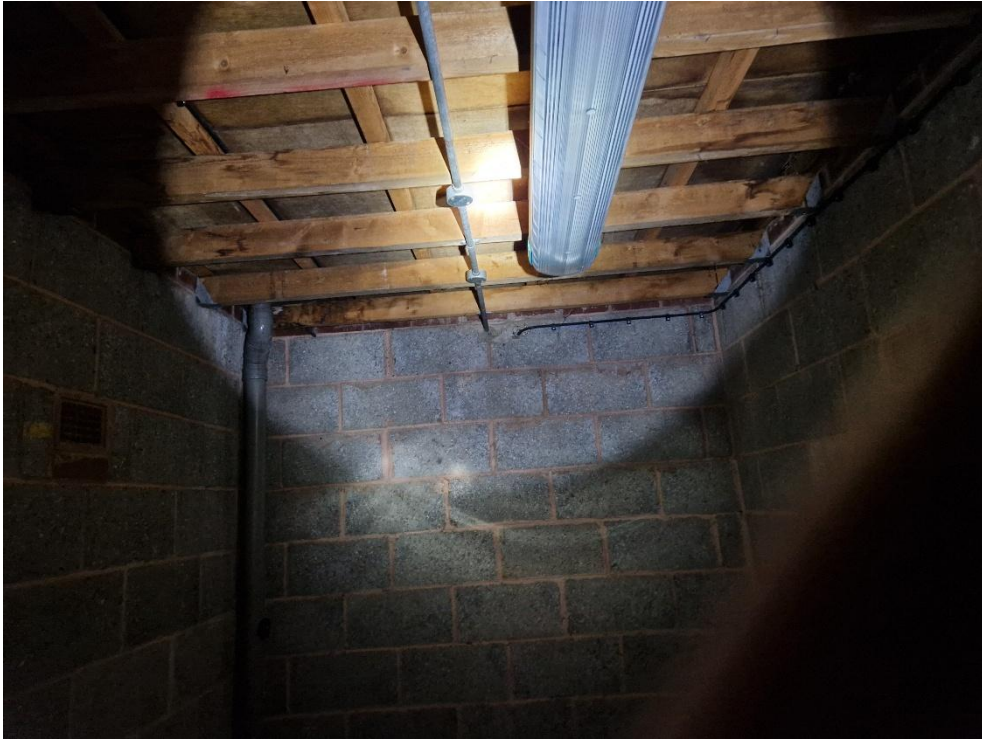
Photograph 15: PRF6 – wooden beams creating gaps and crevices
