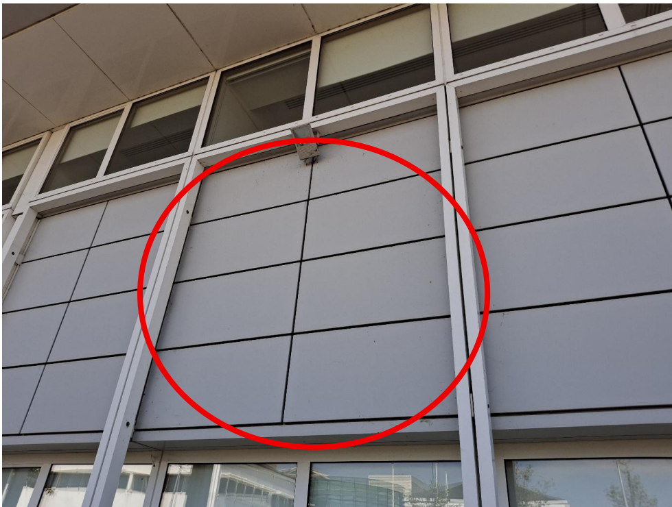
Photograph 10: PRF2 – Gaps leading to suitable sized space behind cladding (northern aspect of B2)
