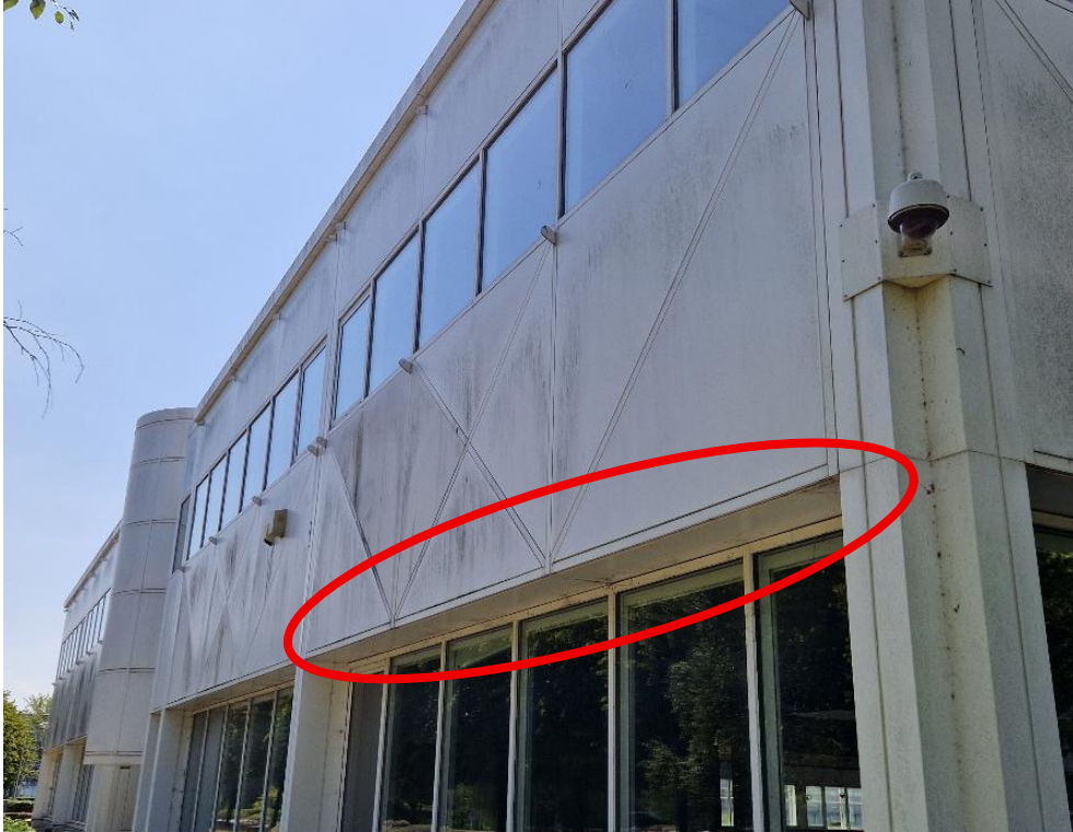
Photograph 11: PRF2 – Gaps leading to suitable sized space behind cladding (southern aspect of B1)
