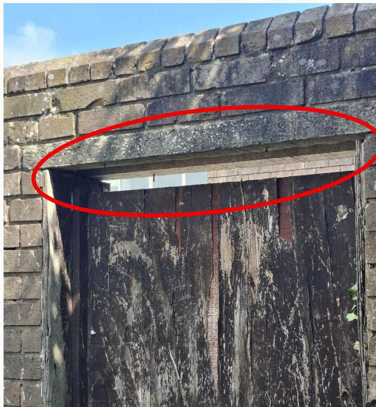
Photograph 14: PRF5 – Cavities within door frame
