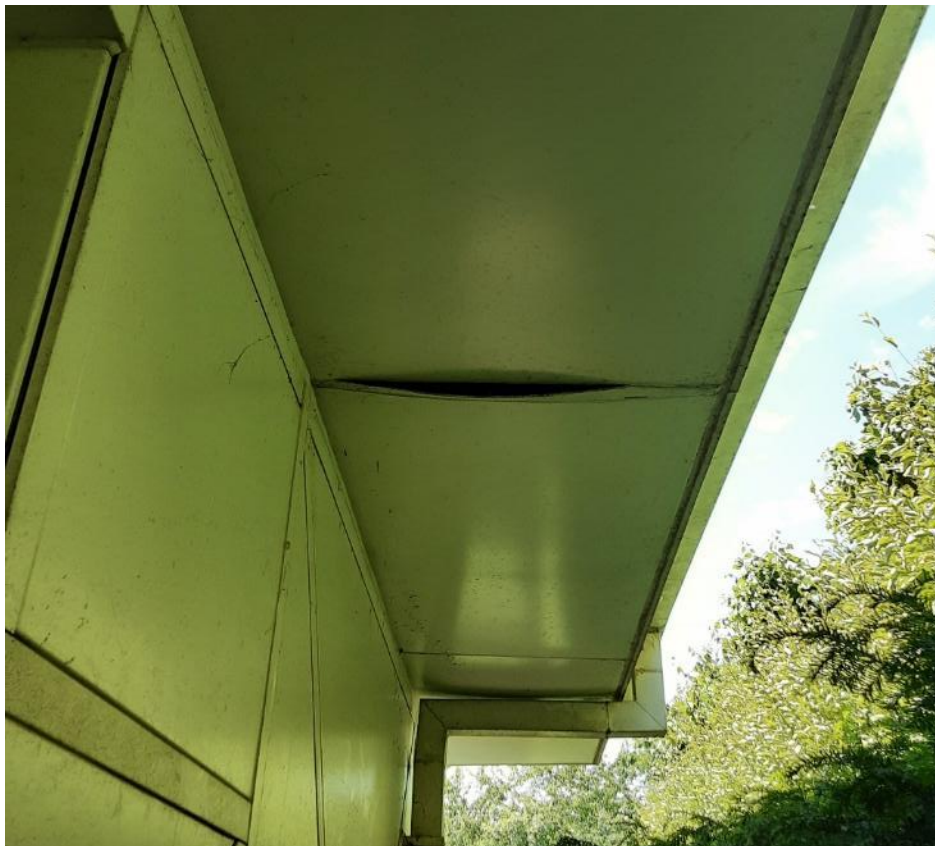
Photograph 8: PRF1 – Gap under soffit
