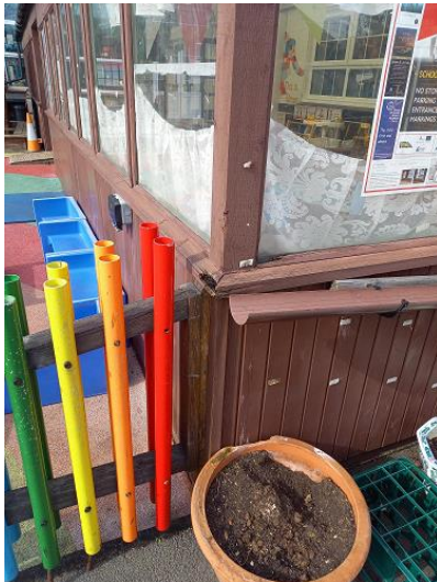
Photo 3 lean to construction rot
