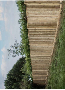
Example of closed boarded fencing
