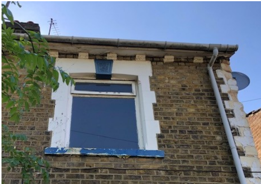
Fig. 28. The degraded stone quoins in the front façade (photo provided by Jordan Wang).
