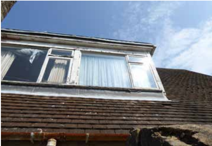
Upgrade/maintenance required to dormers and roof
