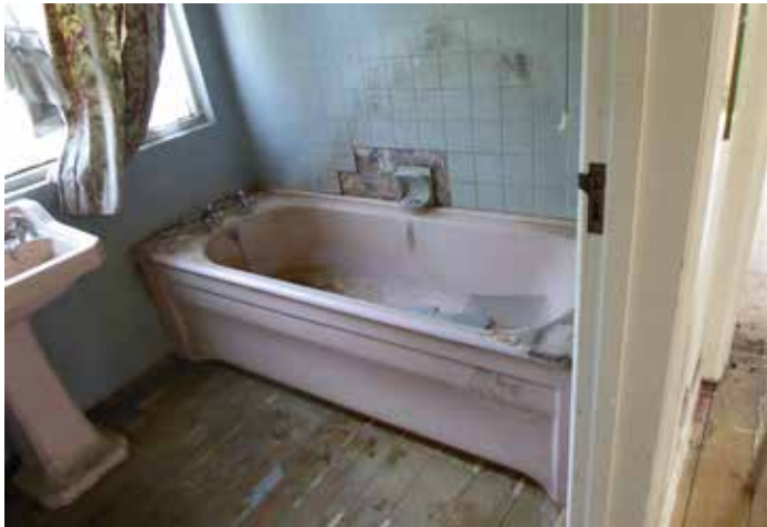
Internal overhaul required
