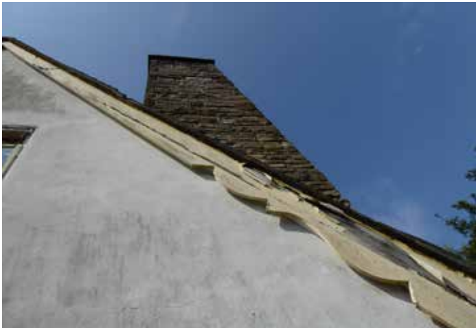
Upgrade/maintenance required to gable end barge boards
