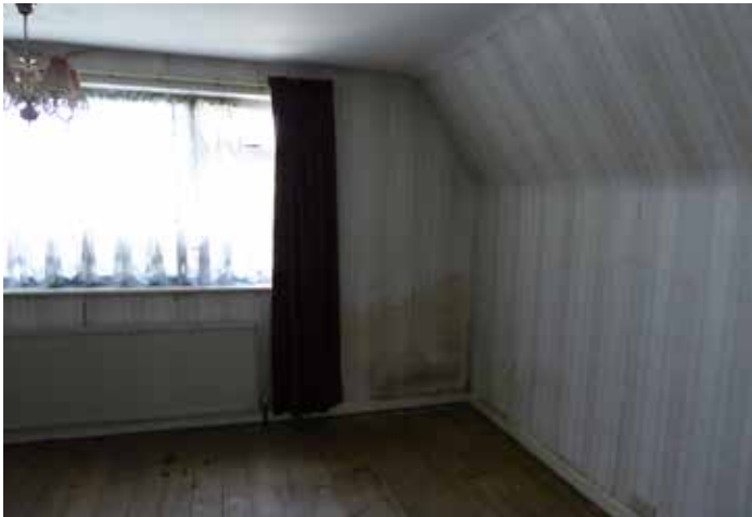
Dampness and damage to rear bedroom
