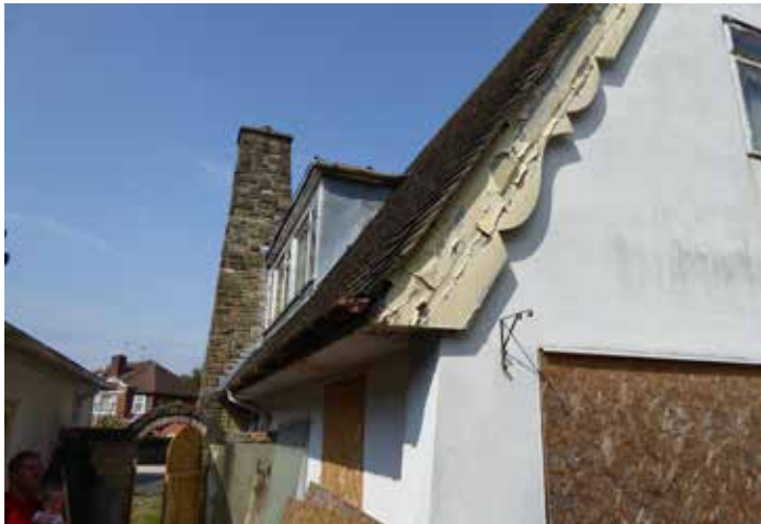
Upgrade/maintenance required to eaves (soffit and fascia)
