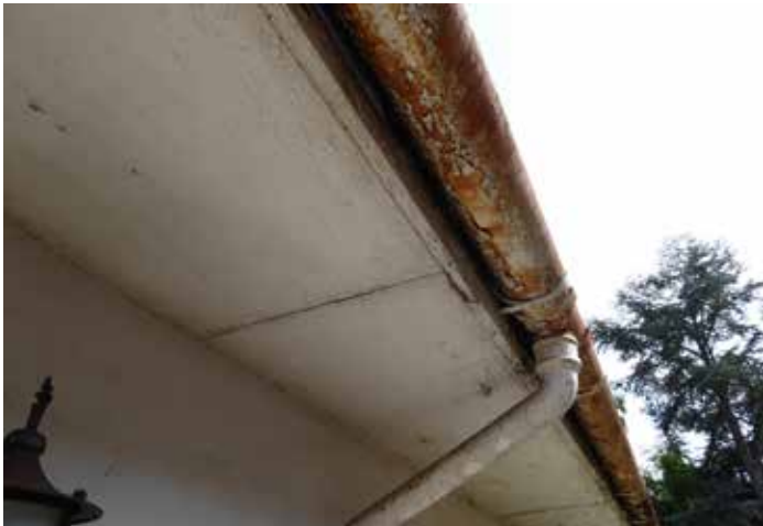
Upgrade/maintenance required to rainwater goods
