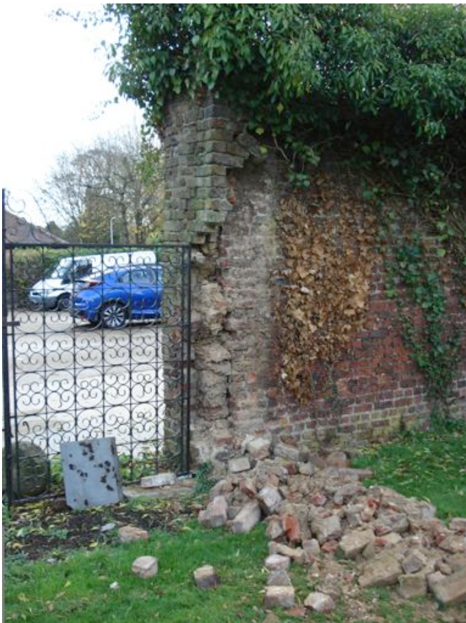
West face of pier following collapse
