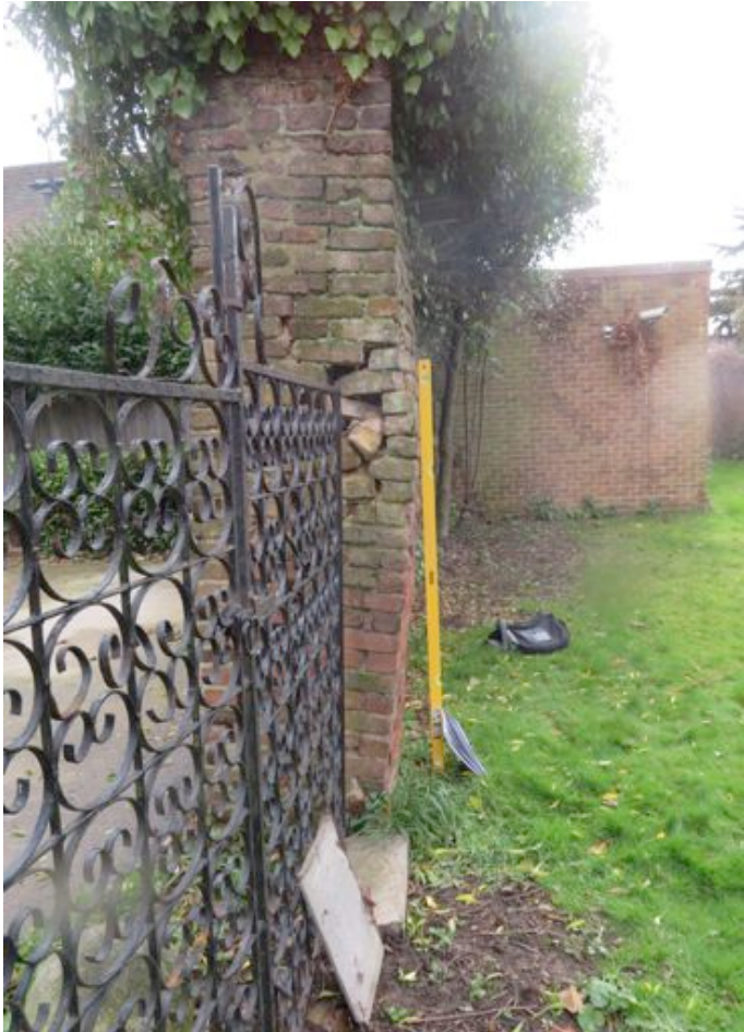
North face of pier prior to collapse. Spirit level is set plumb.
