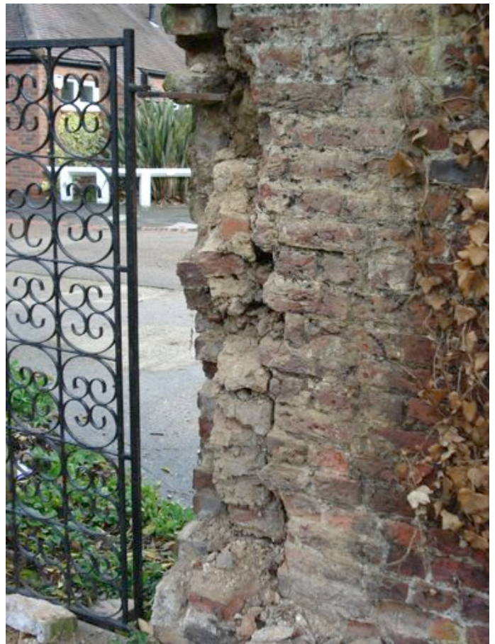
West side of pier following collapse. Note the brick rubble core within the wall and the continuation of the pattern of holes in the brickwork into this area.
