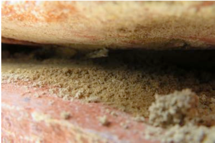
Mortar joint re-opened to show metal tie.
