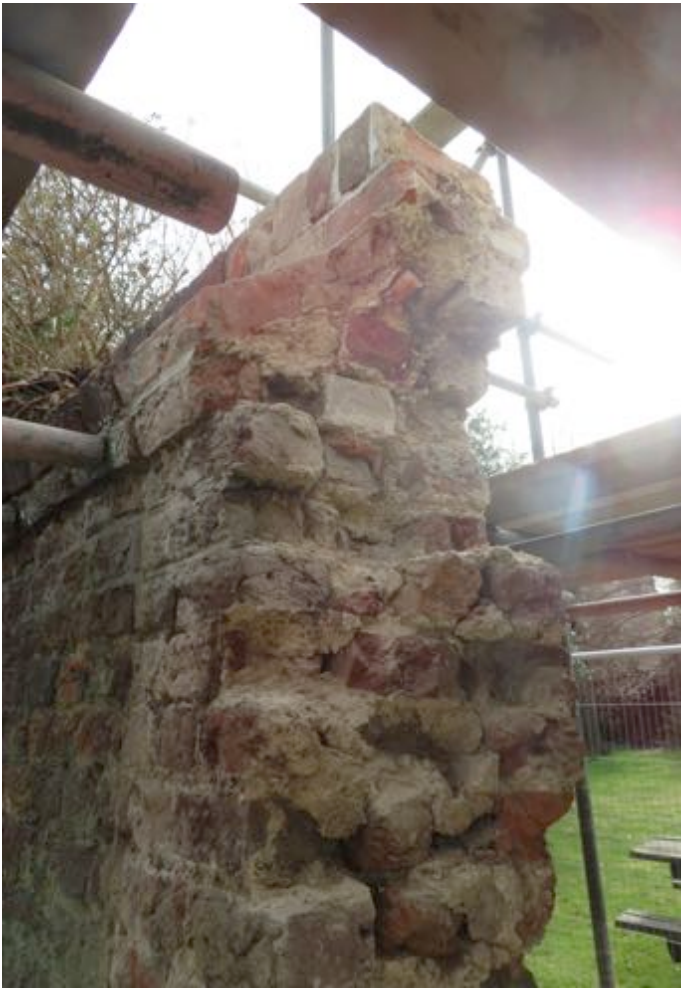
Exposed end of original wall after collapse.
