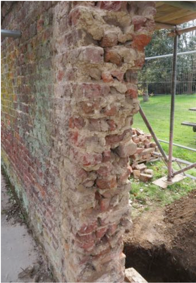
Exposed end of original wall after collapse.
