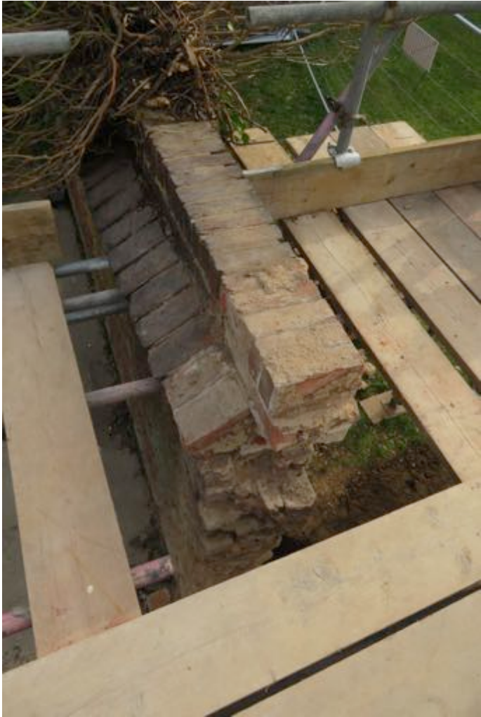
Top of original wall after collapse.
