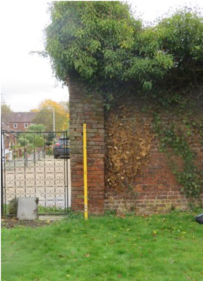
West face of pier prior to collapse. Spirit level is set plumb.
