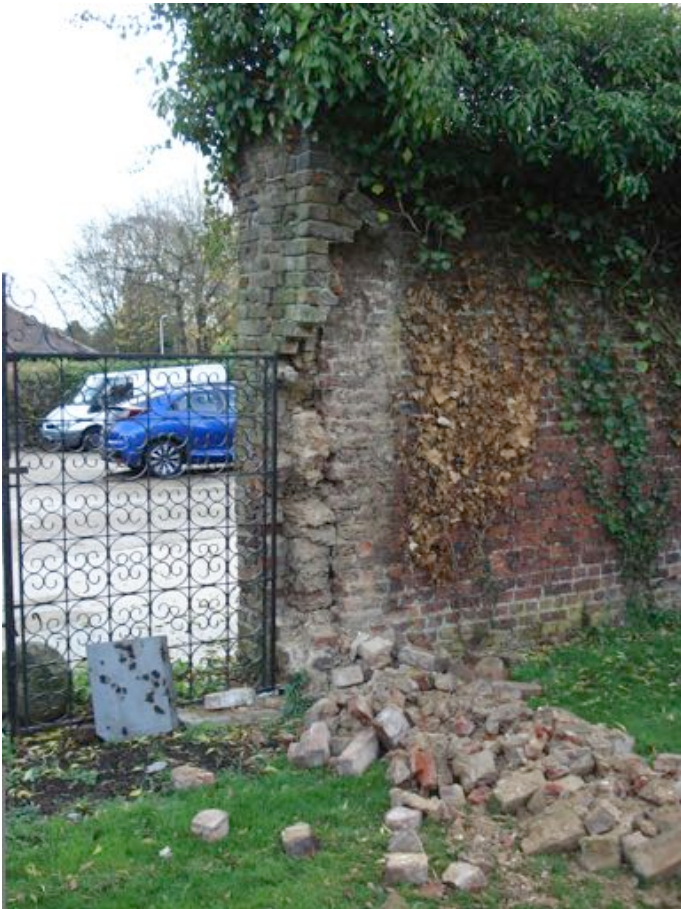
West face of pier following collapse
