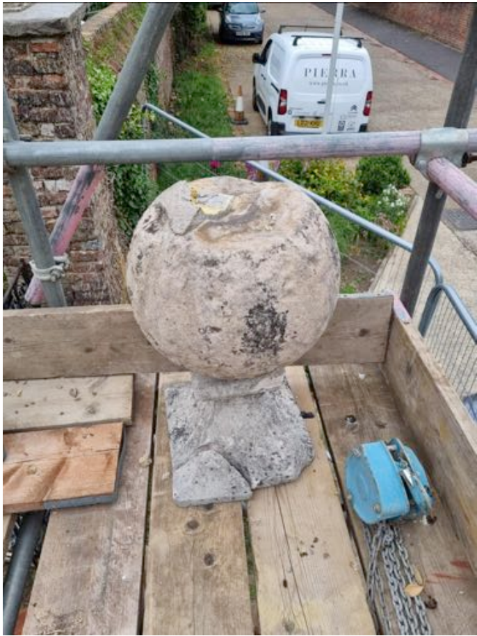
Ball cap prior to repair.
