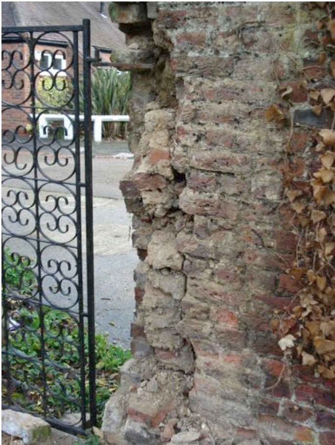
West side of pier following collapse. Note the brick rubble core within the wall and the continuation of the pattern of holes in the brickwork into this area.
