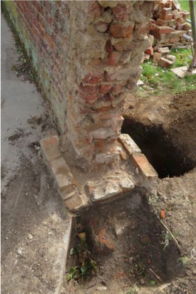
Base of original wall after collapse.
