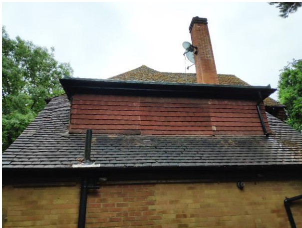
Plate 3.5: Lifted Tiles on Sloped Roof
