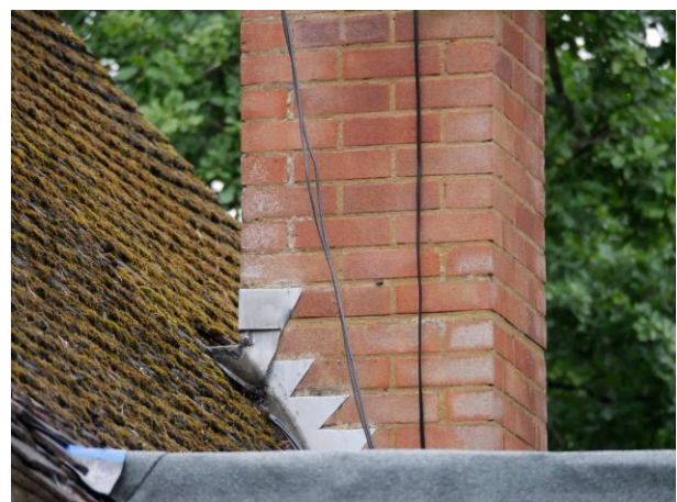
Plate 3.8: Lifted Flashing around Chimney
