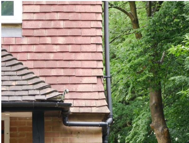
Plate 3.9: Damaged Hanging Tile
