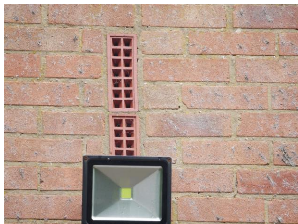
Plate 3.12: Vents – Unsuitable for Bats
