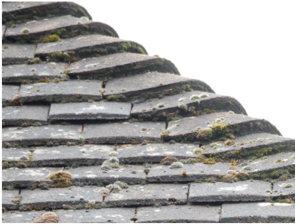
Plate 3.3: Lifted Tiles on Main Roof
