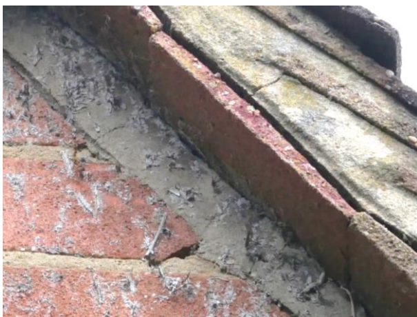
Plate 3.11: Damaged Mortar on Gable Brickwork
