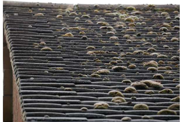
Plate 3.4: Lifted Tiles on the Pitched Gable and Damaged Ridge Tile
