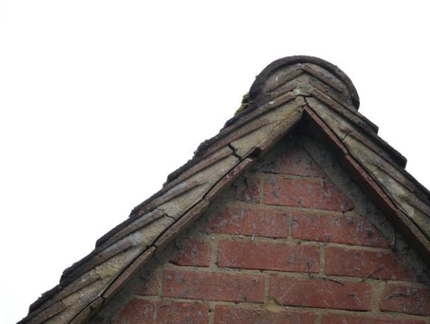
Plate 3.7: Damaged Mortar on Gable
