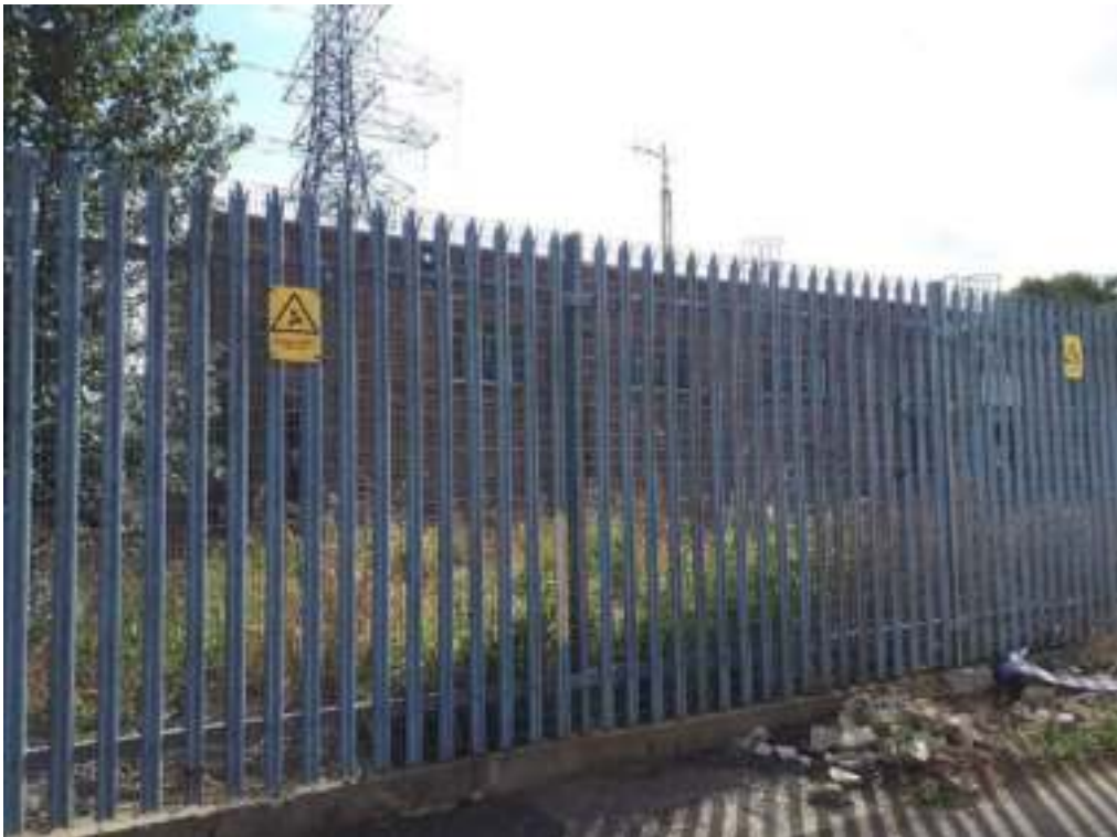
Plate 3: Electricity substation located on Stanwell New Road.
