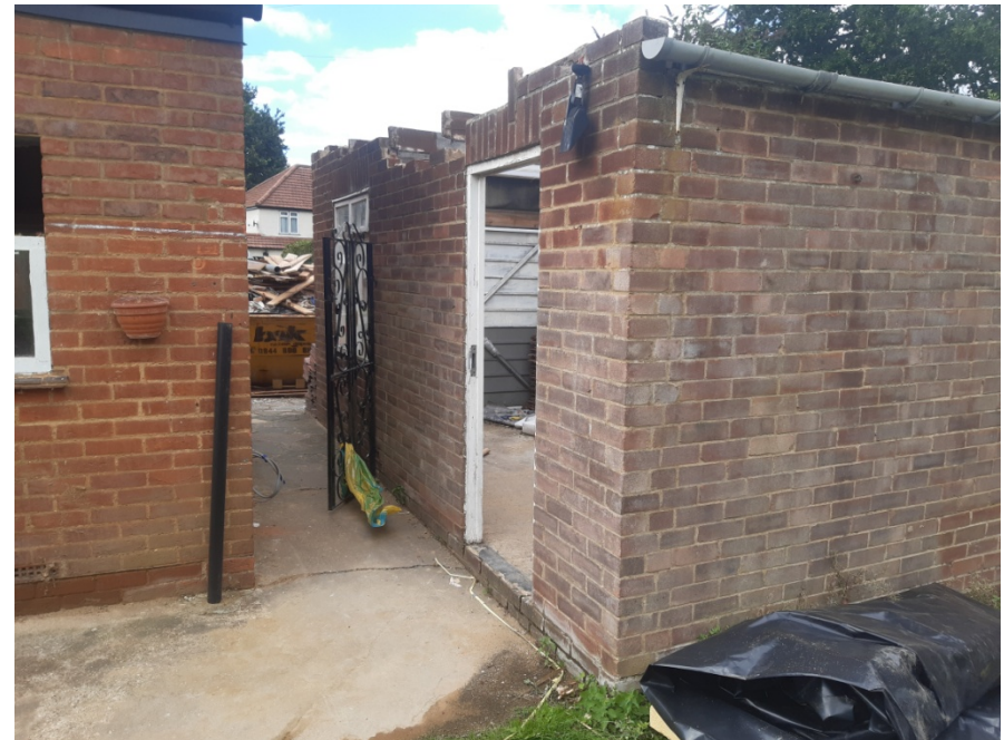
Above: dilapidated garage to be demolished.
