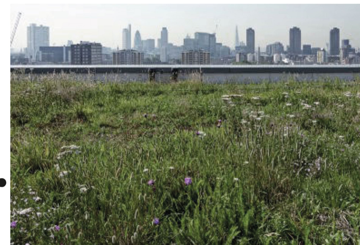
6. GREEN ROOF Intensive Green Roof with deep growing substrate and biodiverse planting of grasses, herbaceous and shrub planting.
