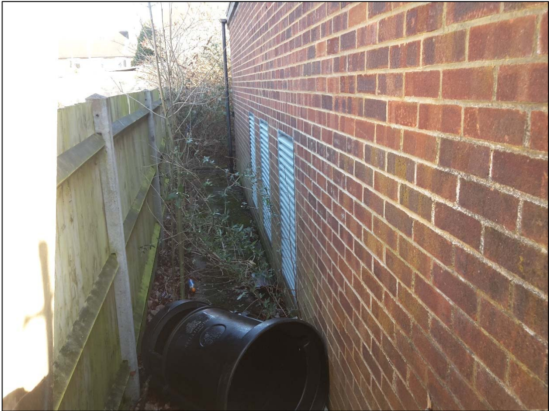
Photograph 7 – Cooling vents adjacent to the western boundary of the site.
