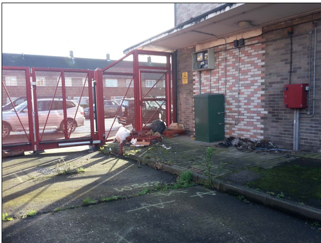
Photograph 4 – Electricity fuse boxes adjacent to the north eastern site entrance.
