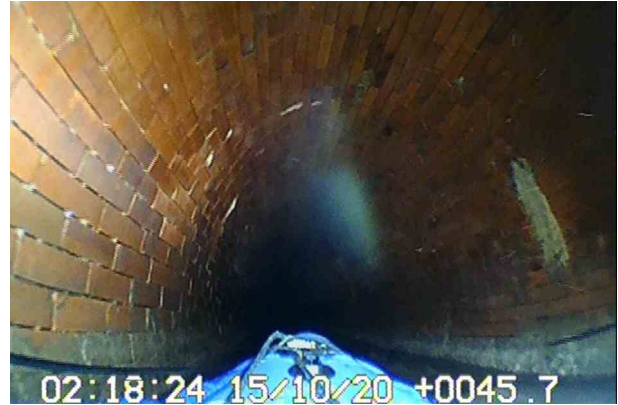
2, 45.80 m Attached deposits, encrustation from 2 o'clock to 4 o'clock, 5% cross-sectional area loss, SUGGESTS SLIGHT INFILTRATION
