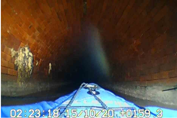
5, 159.20 m Attached deposits, encrustation from 8 o'clock to 10 o'clock, 5% cross-sectional area loss, SUGGESTS SLIGHT INFILTRATION
