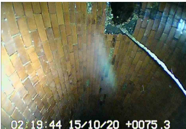
3, 75.30 m Connection other than junction at 12 o'clock, diameter: 300mm, LAMP HOLE (RAG HANGING)
