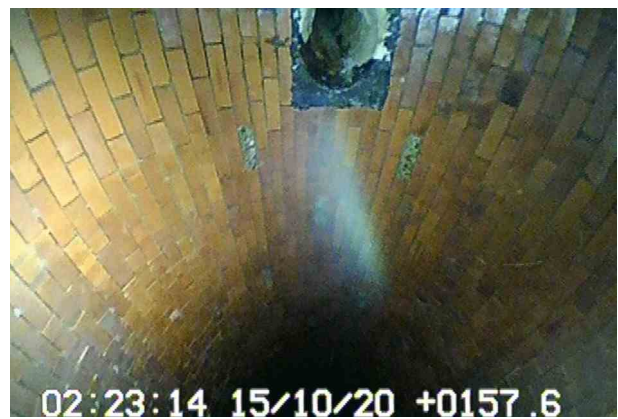
4, 157.60 m Connection other than junction at 12 o'clock, diameter: 300mm, LAMP HOLE
