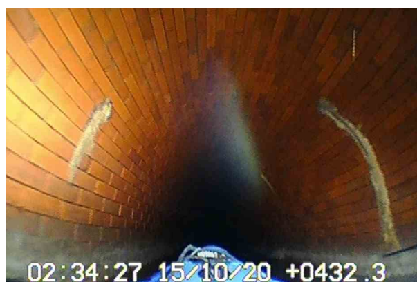
14, 432.20 m Attached deposits, encrustation from 1 o'clock to 4 o'clock, 5% cross-sectional area loss, SUGGESTS SLIGHT INFILTRATION
