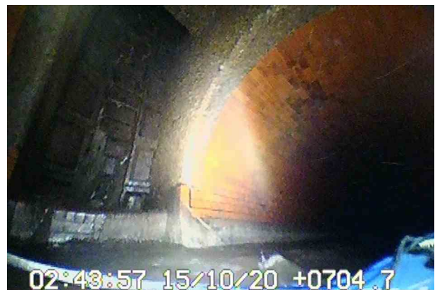
20, 704.70 m Finish node type, manhole, reference number: TQ10794101
