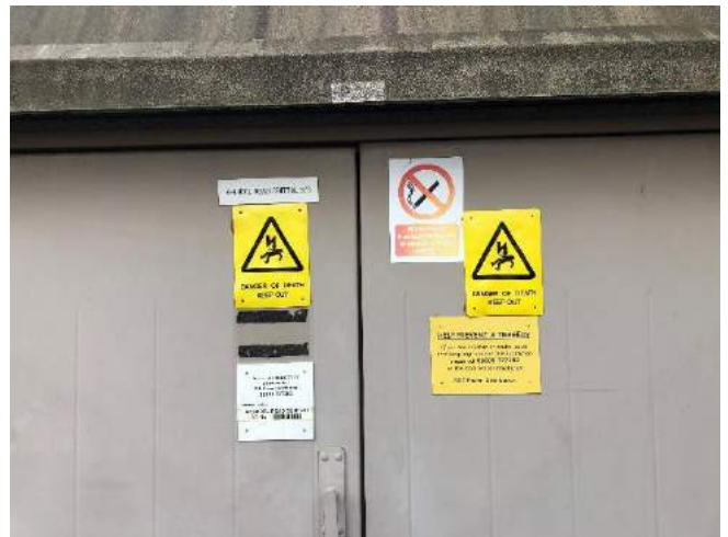
Electricity sub-station housing, in rear yard
