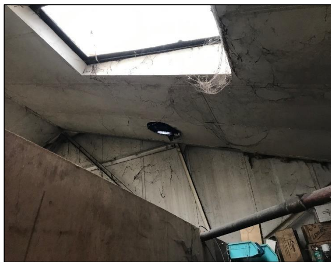
Appendix B Figure 26: Ceiling and wall join, lots of cobwebs
