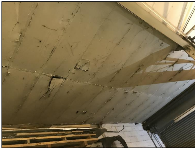
Appendix B Figure 25: : Damaged ceiling boards allowing for potential access into ceiling cavity
