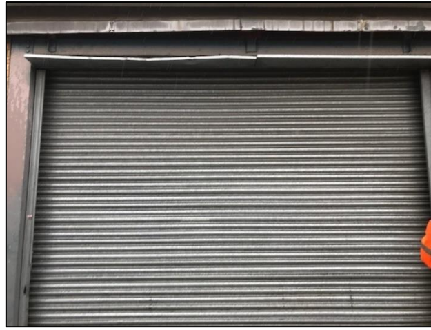
Appendix B Figure 51: Crevice created between the top of the roller door and the east facing wall
