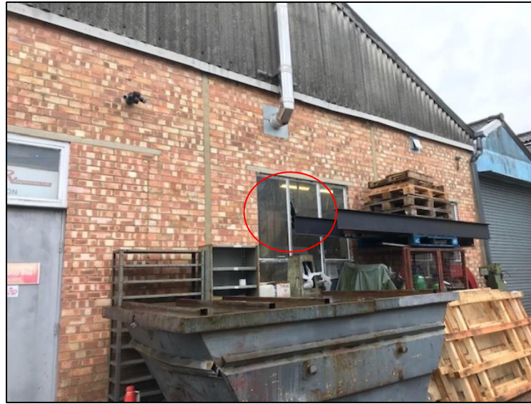
Appendix B Figure 19: Broken front window circled in red
