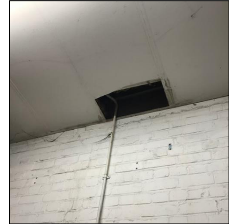
Appendix B Figure 44: Gaps in the ceiling tiles allows for access points between the roof and the ceiling cavity.
