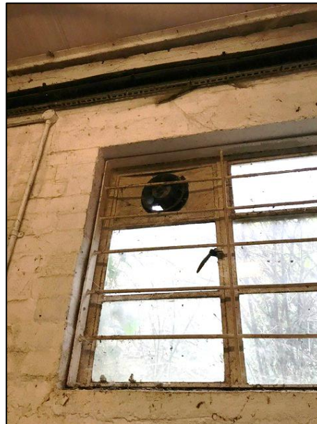
Appendix B Figure 46: Potential access route via the broken fan in a window on the bottom floor. The access hole opens out into the woodland.
