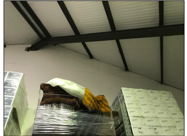
Appendix B Figure 57: Wooden beams on the roof, a cavity is created where the beam meets the unit wall.
