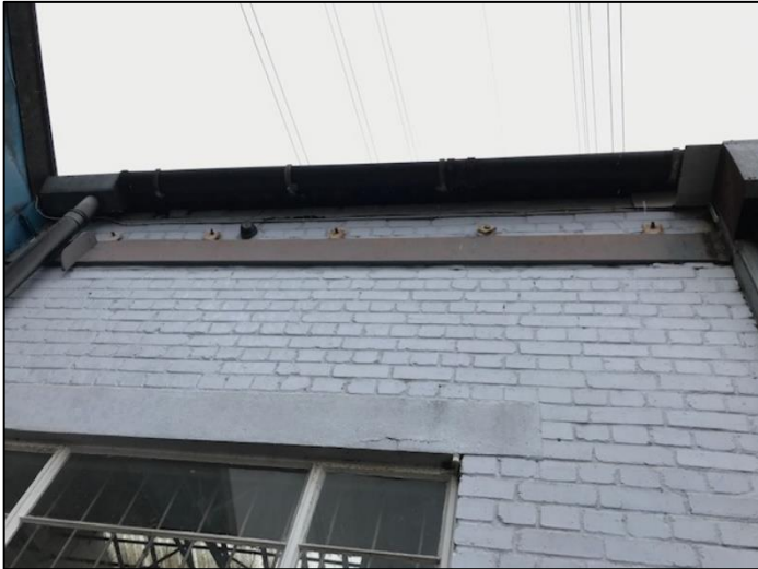
Appendix B Figure 30: Crevice between wall and guttering
