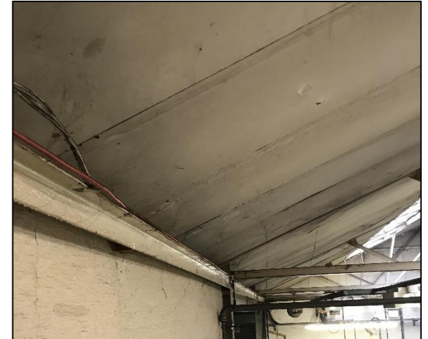
Appendix B Figure 24: Potential crevices in wall and ceiling join
