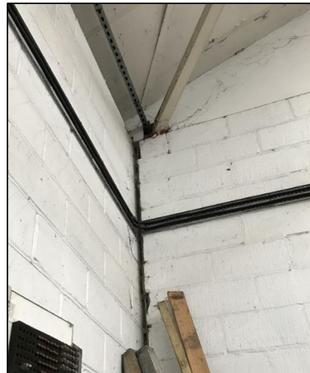
Appendix B Figure 33: Crevices between wall joins in the corners of the room
