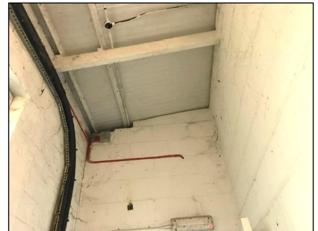
Appendix B Figure 47: Crevices created around the wooden beams when they meet the wall in the switchboard room.
