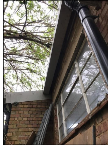
Appendix B Figure 39: Potential wall roof gap below guttering
