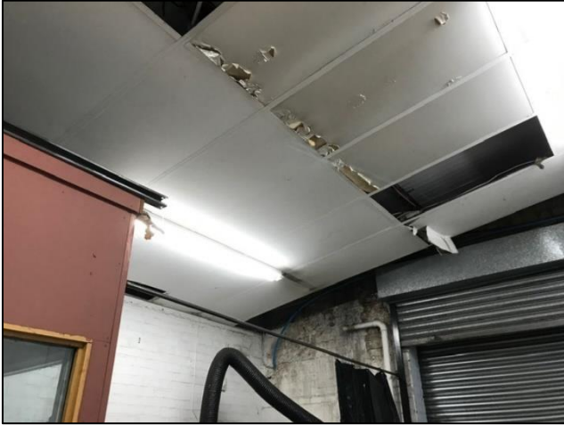
Appendix B Figure 42: Unit E degraded ceiling boards allowing access to cavity between ceiling and roof
