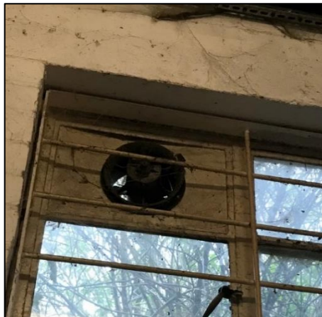
Unit E, hole in fan in ground floor window
