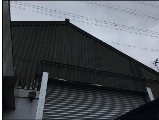
Appendix B Figure 11: Crevice between roller door and roof
