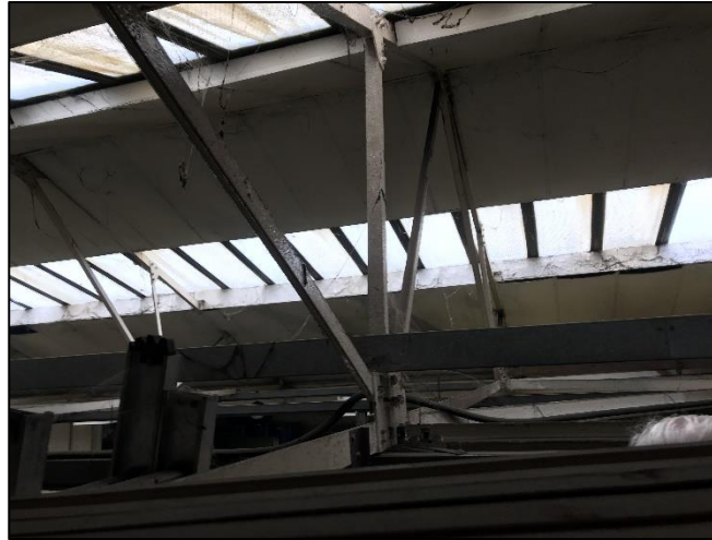
Appendix B Figure 23: Warehouse ceiling has cobwebs
