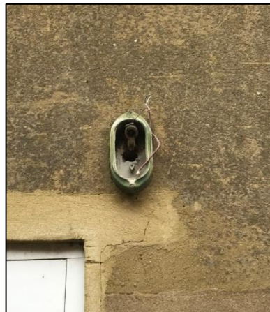
Unit B, potential hole in external wall below roof
