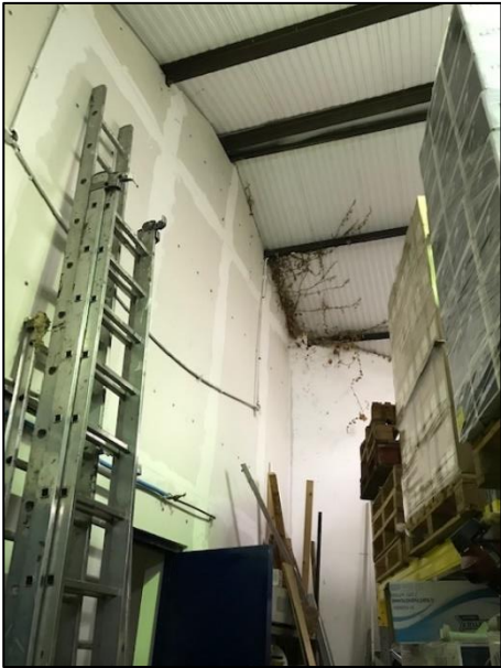
Appendix B Figure 55: Ivy (Hedera helix) on the southwest corner, entering through a wall-roof gap.
