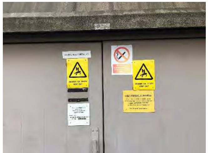
Electricity sub-station housing, in rear yard
