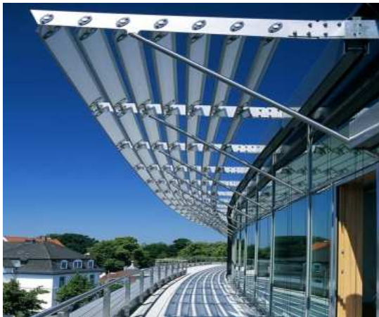
Figure 3: Solar PV Louvres on the South Façade
