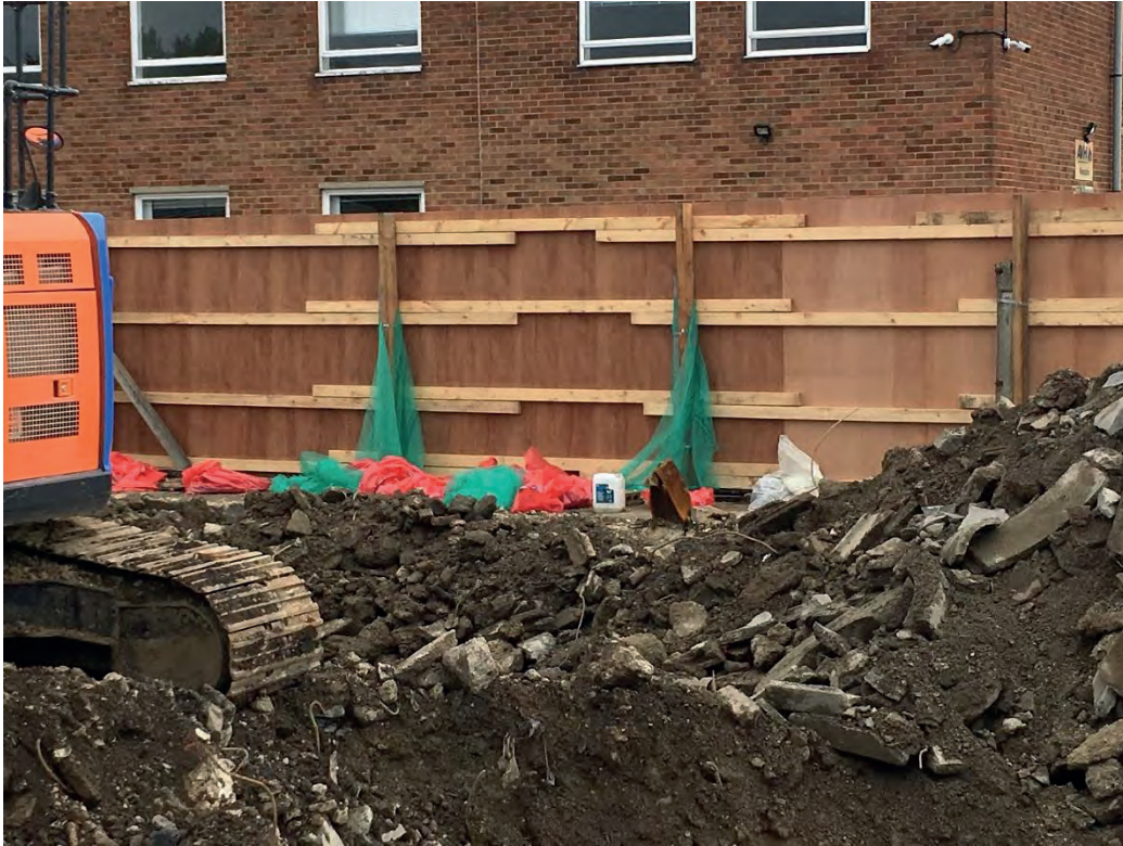
Fig 5. Asbestos kept in special red asbestos bags on Site.
