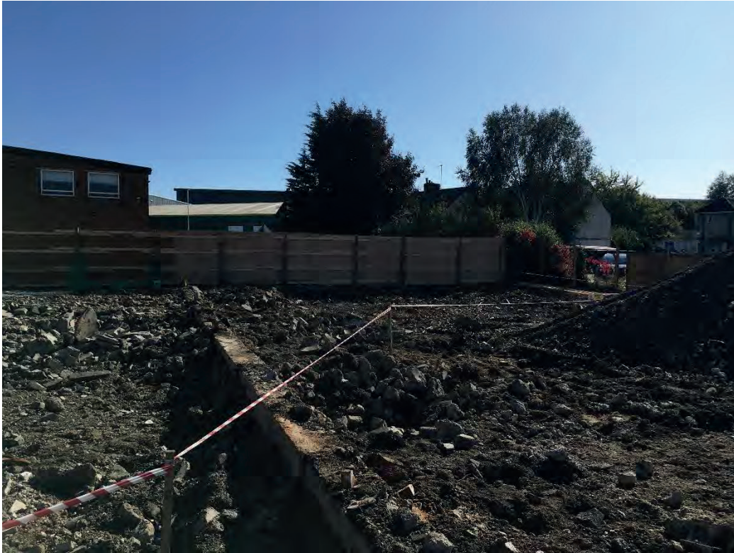
Fig 3. Crushing area to the east of the Site. Asbestos found.
