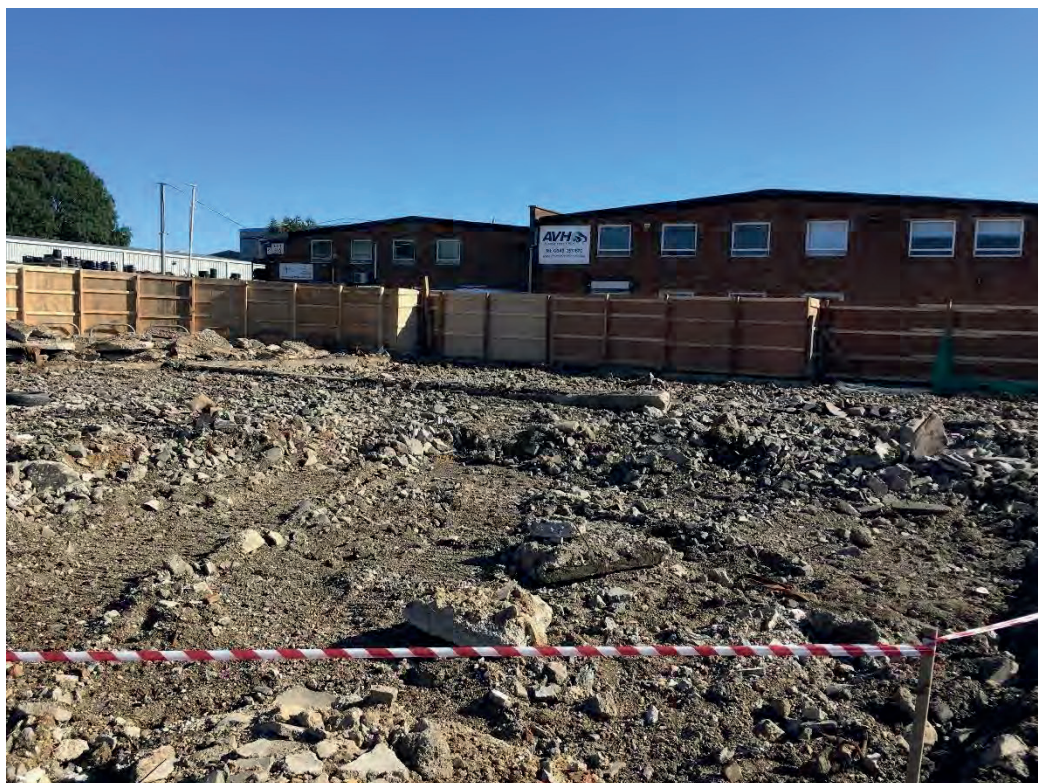
Fig 2. Crushing area to the east of the Site. Asbestos found.
