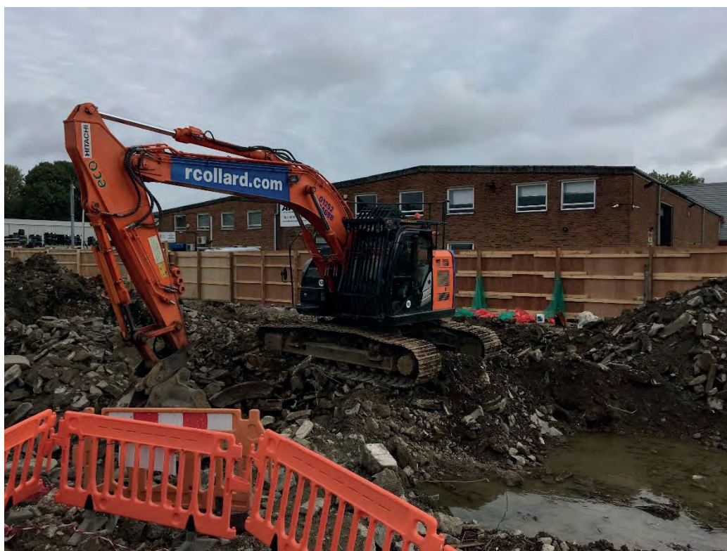
Fig 4. Asbestos area where asbestos specialists were working at the moment that Delta Simons visited the Site.
