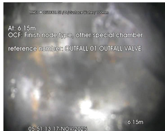
MH01X_64ba4c82-0a89-442b-89d8-16b16120b461_20251114_150607_229.jpg, 00:01:20, 6.15 m Finish node, other special chamber, reference: OUTFALL 01, OUTFALL VALVE
