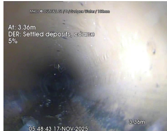
MH01X_5d0f0135-f28d-4204-93b7-4b86a68ea43d_20251114_150558_942.jpg, 00:00:41, 3.36 m Settled deposits, coarse, 5% cross-sectional area loss
