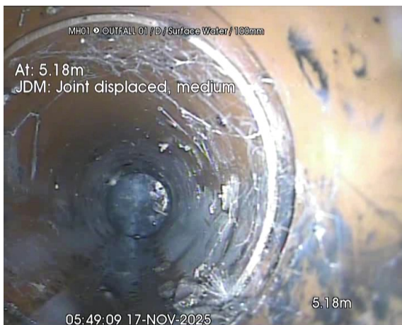
MH01X_9ebad77c-1627-45fe-aa61-7b387f23d6e7_20251114_150602_827.jpg, 00:01:01, 5.18 m Joint displaced, medium
