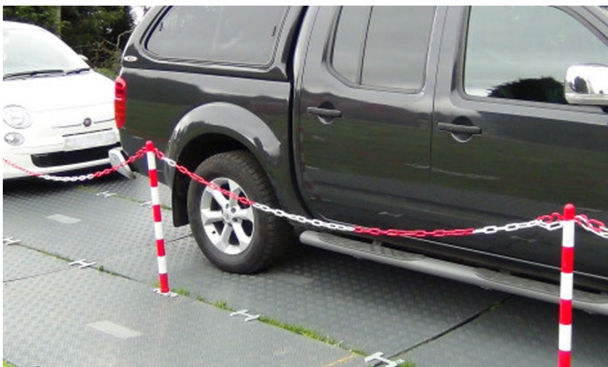
Fig. 3 Ground Guards Lite Track provide a suitable surface for vehicles and light construction plant over the cellular confinement area
