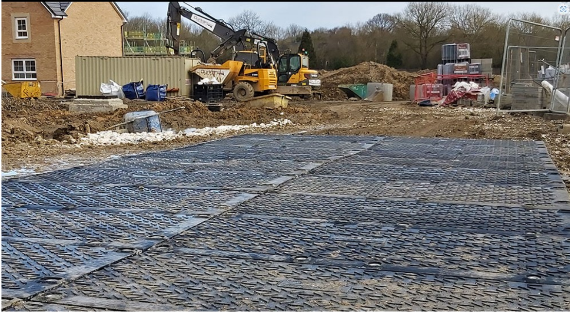
Fig. 3 Ground Guards – Maxi Trak Heavy duty is ideal for the ground protection required here.
