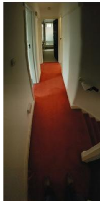
No. 33 Kingsend – Current landing, demonstrating width and lack of light
