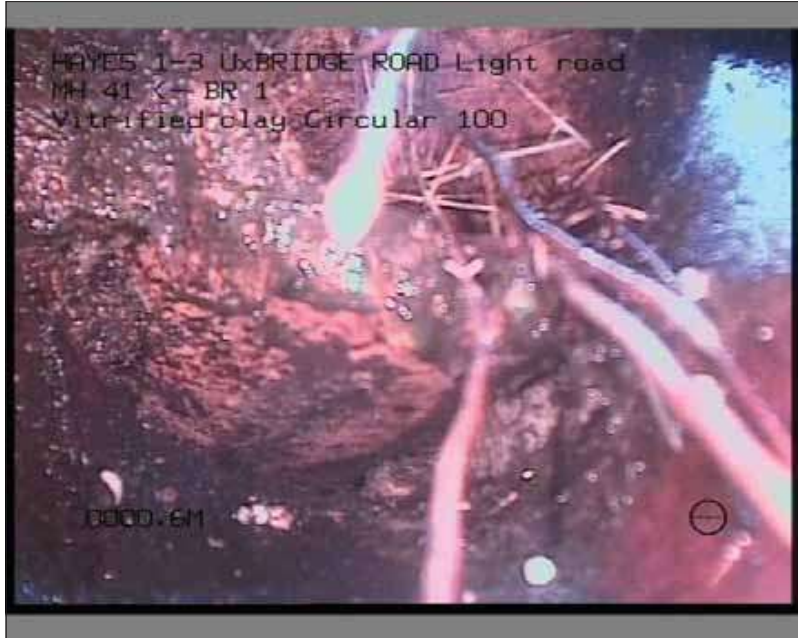
Photo: 68_69_624_A.JPG 0.6m, Roots, mass, 95% cross-sectional area loss
