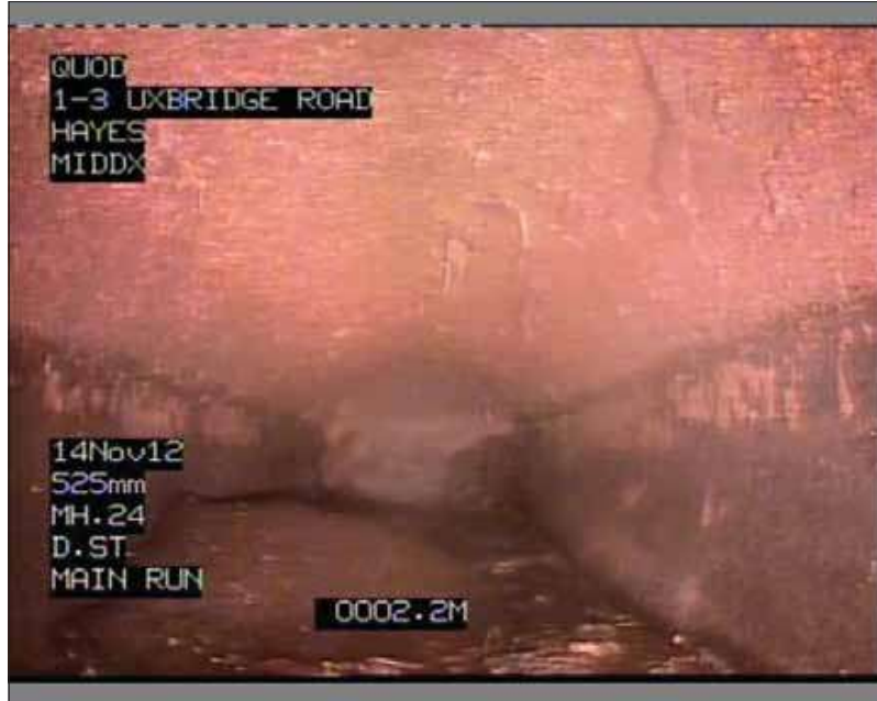
Photo: 53_54_481_A.JPG 2.2m, Debris, 20% cross-sectional area loss
