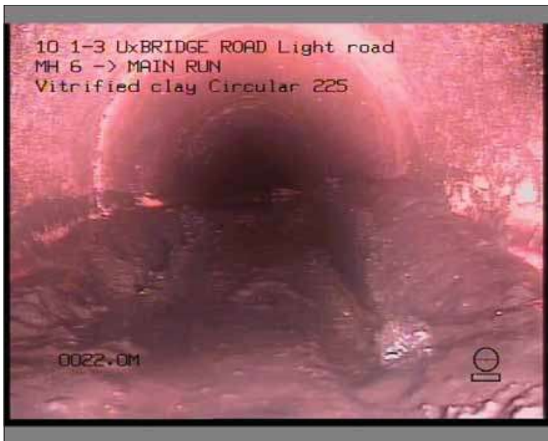
Photo: 19_20_160_A.JPG 21.4m, Debris silt, 30% cross-sectional area loss, Start
