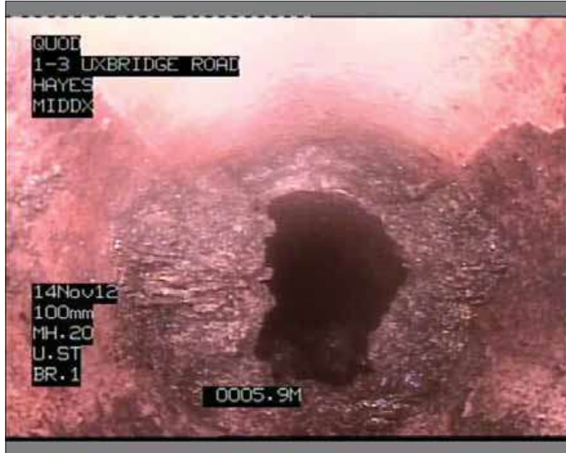
Photo: 44_45_407_A.JPG 5.9m, Survey abandoned Remarks: DUE TO EHJ
