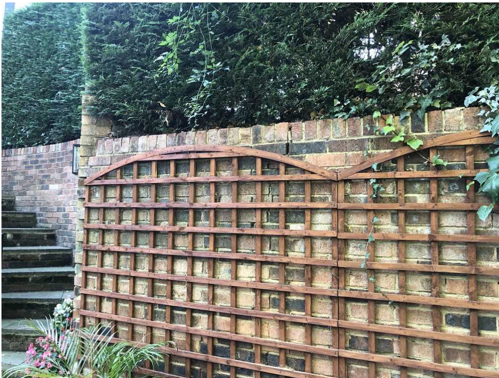
Crack seen in 9 inch brick garden retaining wall. Land level high behind the wall and conifer hedge
