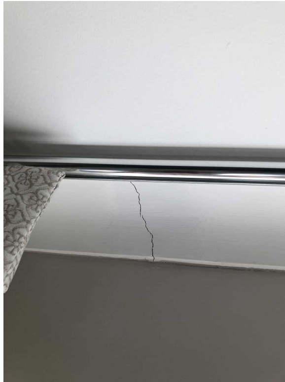
And slight ceiling crack
