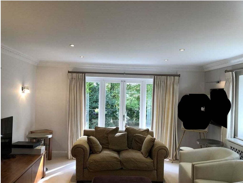
Back elevation bi-fold window corner cracks and cornice line gaps
