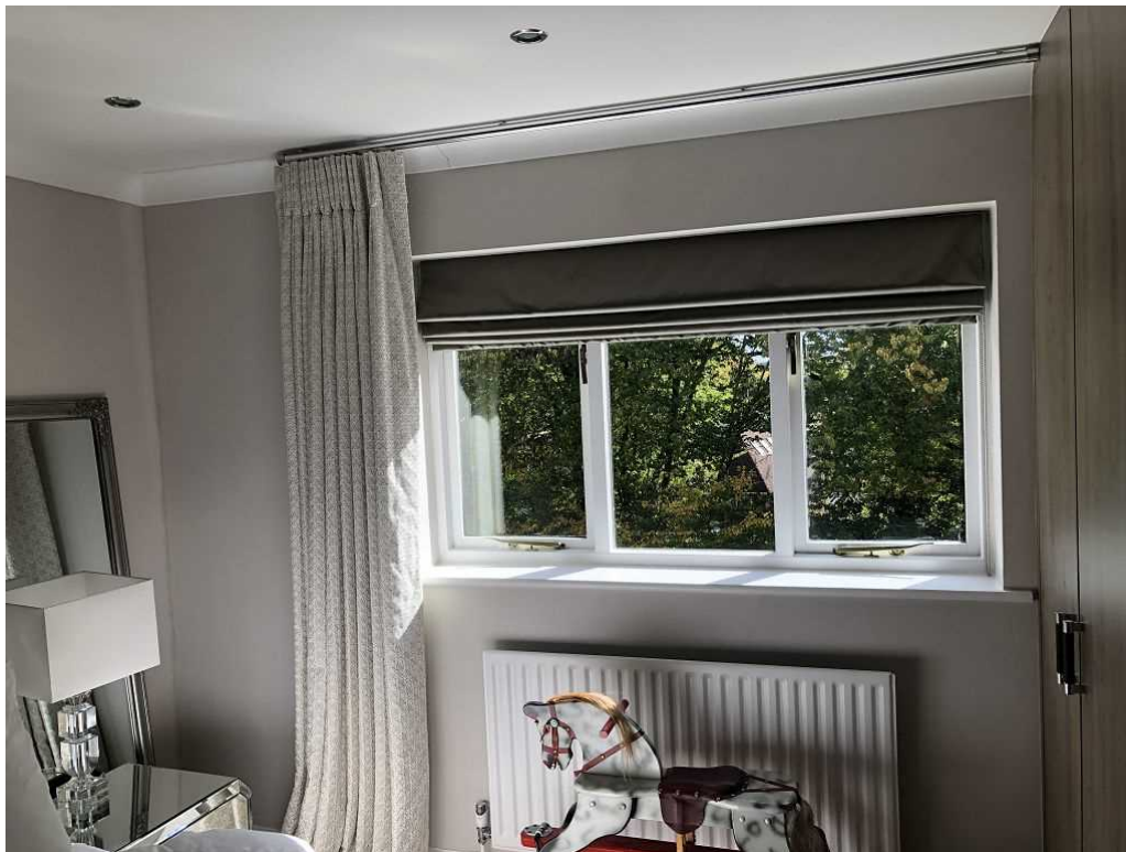
Back left corner bedroom - 1mm crack under sill
