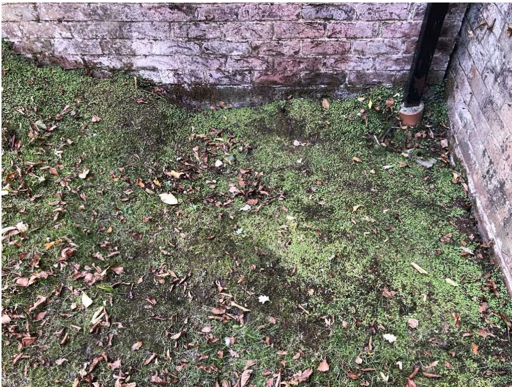
The ground in this corner sunken and very damp but it is a low point
