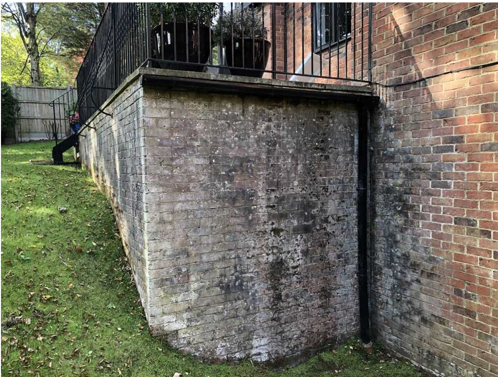
Back raised terrace junction with the main house- large 40mm rotation type gap as described in the engineer report
