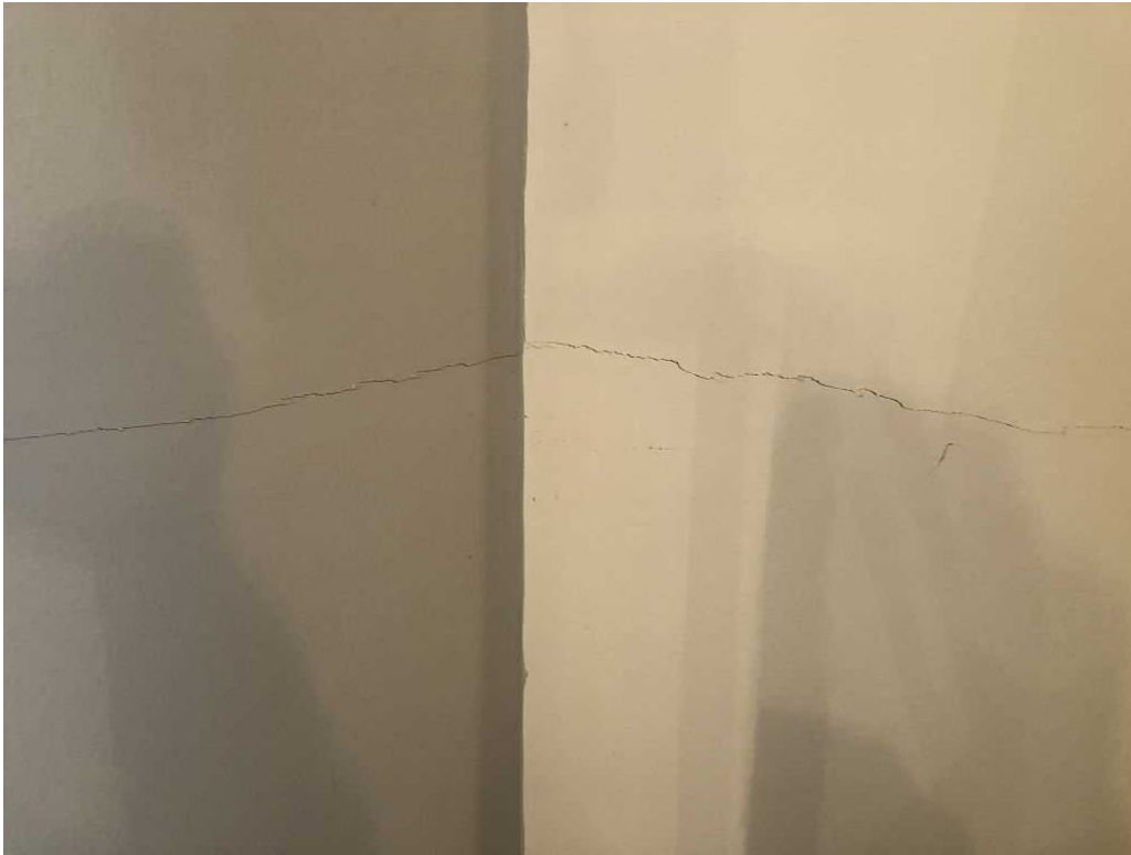
And crack lines in the wall front right corner
