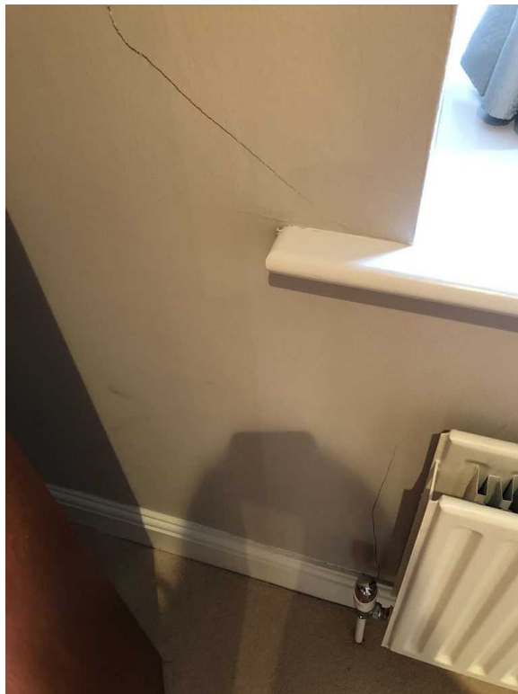
And smaller crack bottom left window corner
