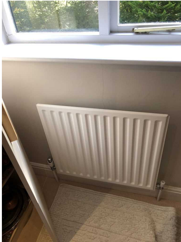
Rear elevation central small bedroom. Crack 1mm under sill and behind radiator
