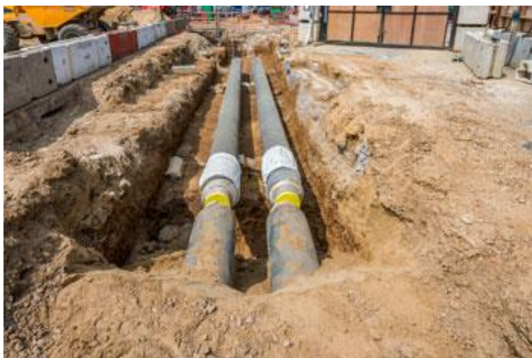
Figure 8. District heating pipework 4
