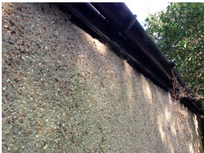
Photograph 9: Small gap behind fascia board on the garage.
