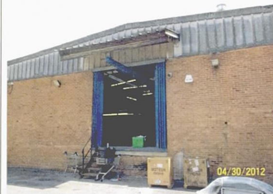
Asbestos Containing Materials
