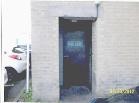
Open access door to neighbouring facility to be secured
