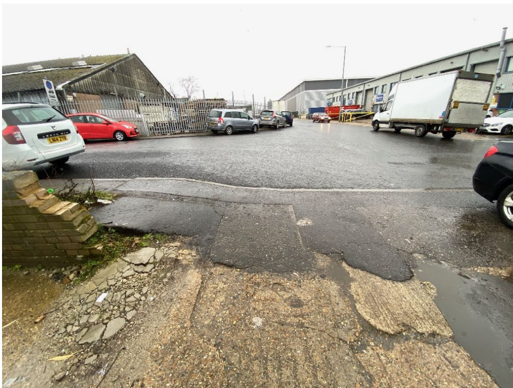
3. View looking north-east from within the front boundary of the application site towards the existing dropped kerb, showing the failing boundary wall.
