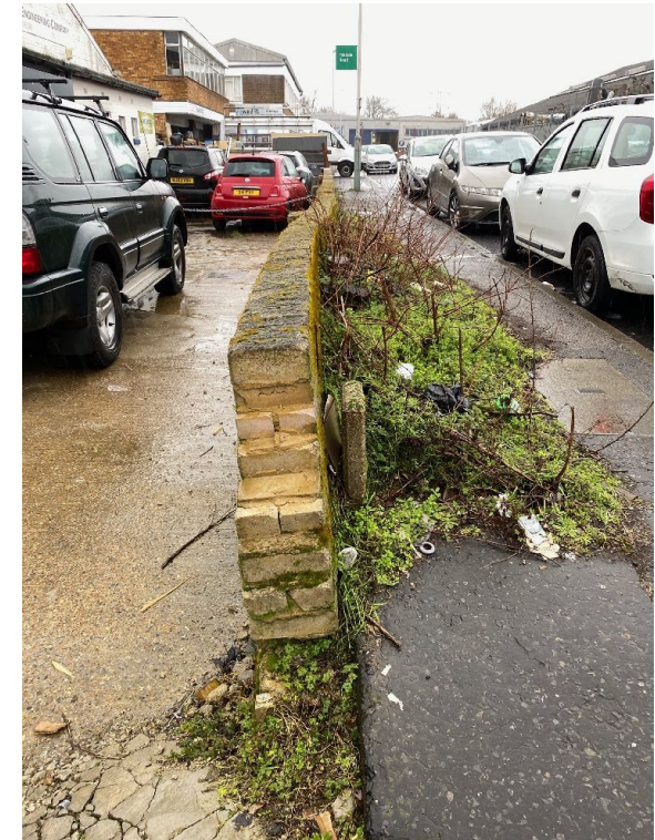
2. View looking north-west showing the front boundary wall, note wall is failing due to tree stump on the pavement.
