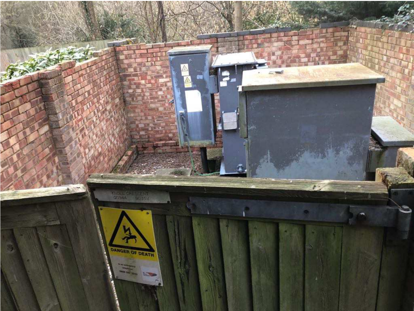
Photo No. 4 to show the fenced-off electric transformer under T1
