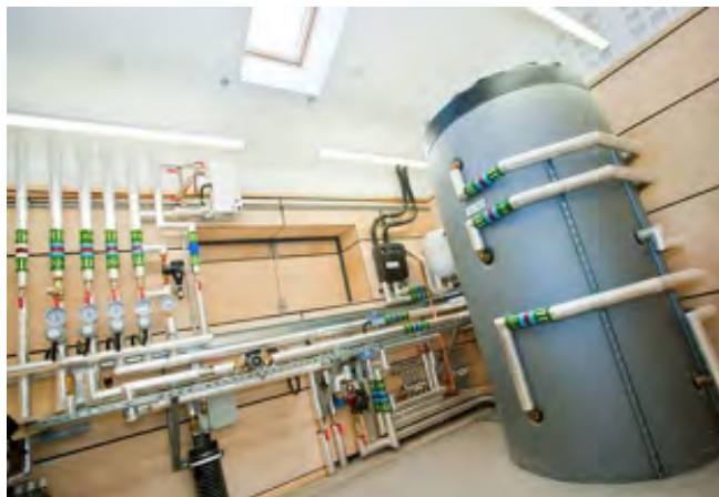
Treco Biomass Boiler
