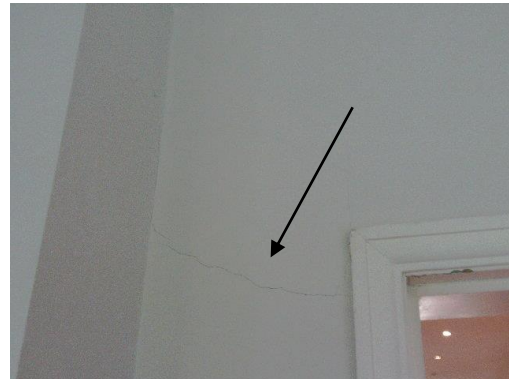
Cracking in rear extension
