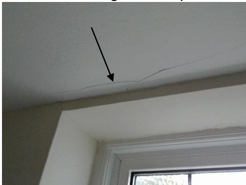
Cracking in w.c.
