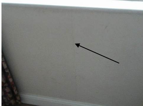
Rucking below half landing flank window
