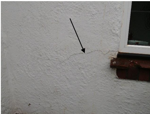
Cracking to right hand flank below w.c. window
