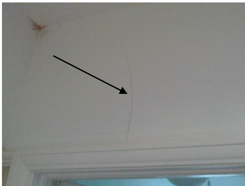
Cracking in hallway
