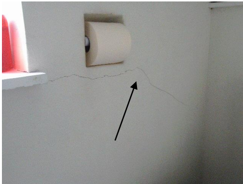
Cracking in w.c.
