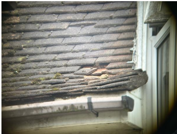
Figure 10. Damaged roof tiles on adjoining 11 Beech Avenue
