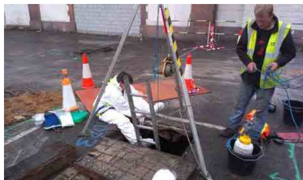
Confined space entry setup
