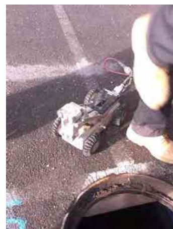
Pipework in duct
