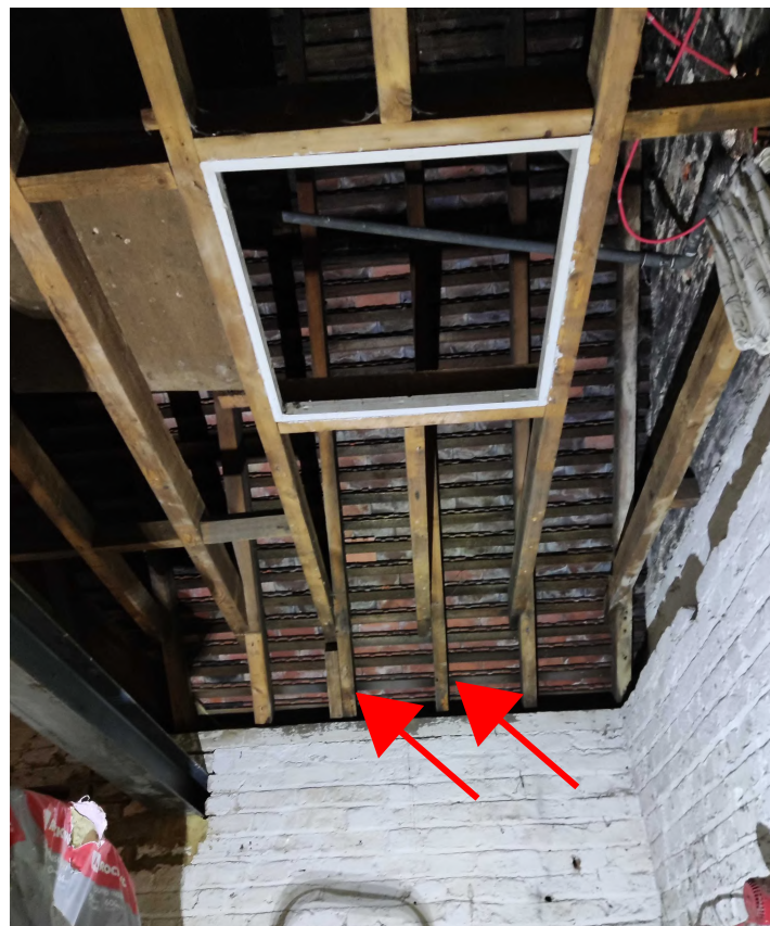
Rafters at frame No.66 and 67 are decayed and needs replacement.
