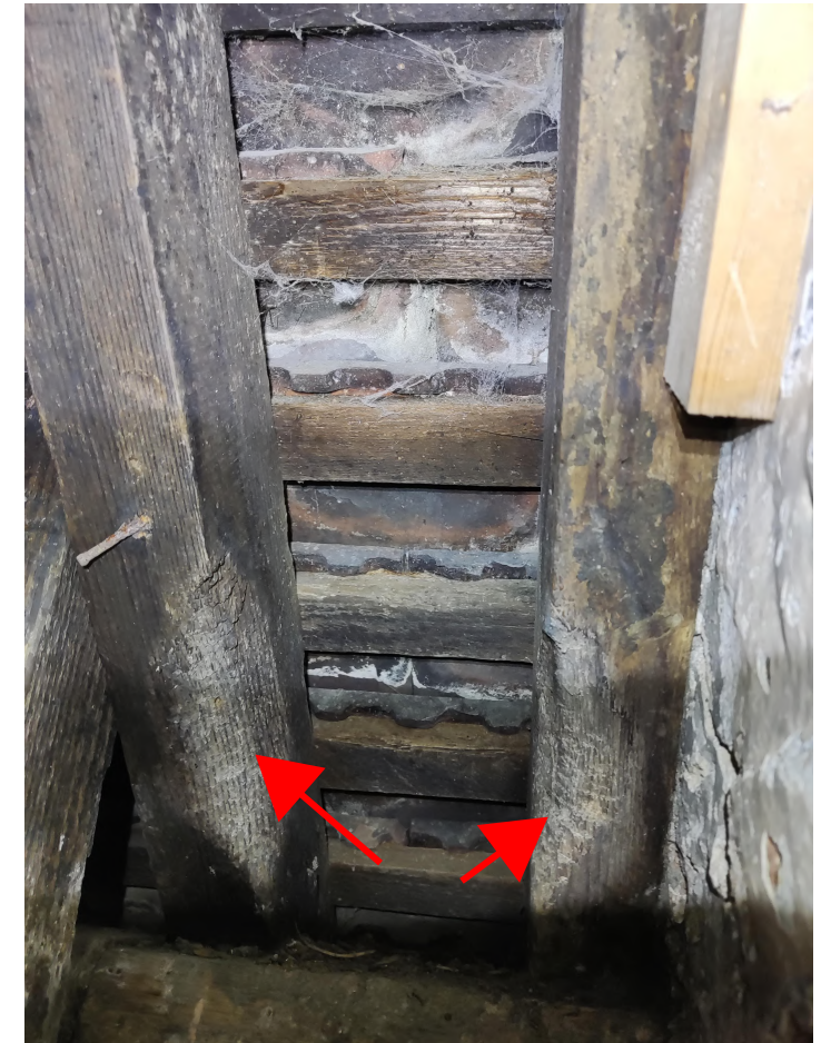
Roof Frame 45 and 46 decayed and should be replaced.
