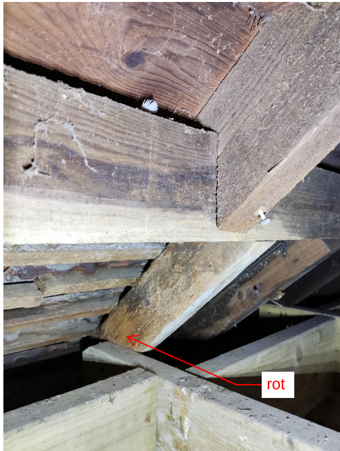
Rafter at frame No.39 is decayed and needs replacement.
