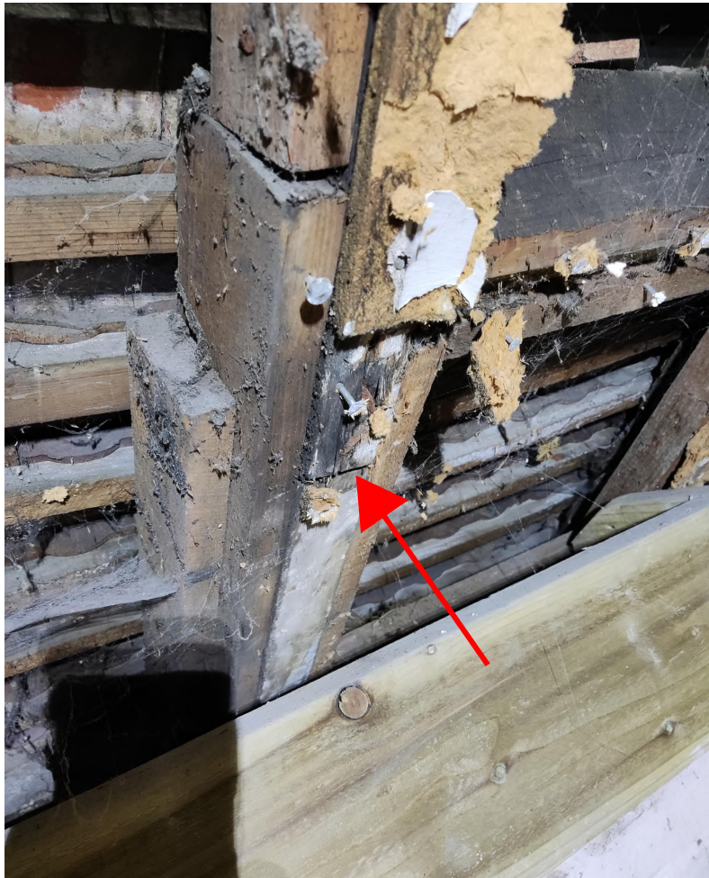
Poor repair to roof rafter at frame No.14. The rafter to be replaced.
