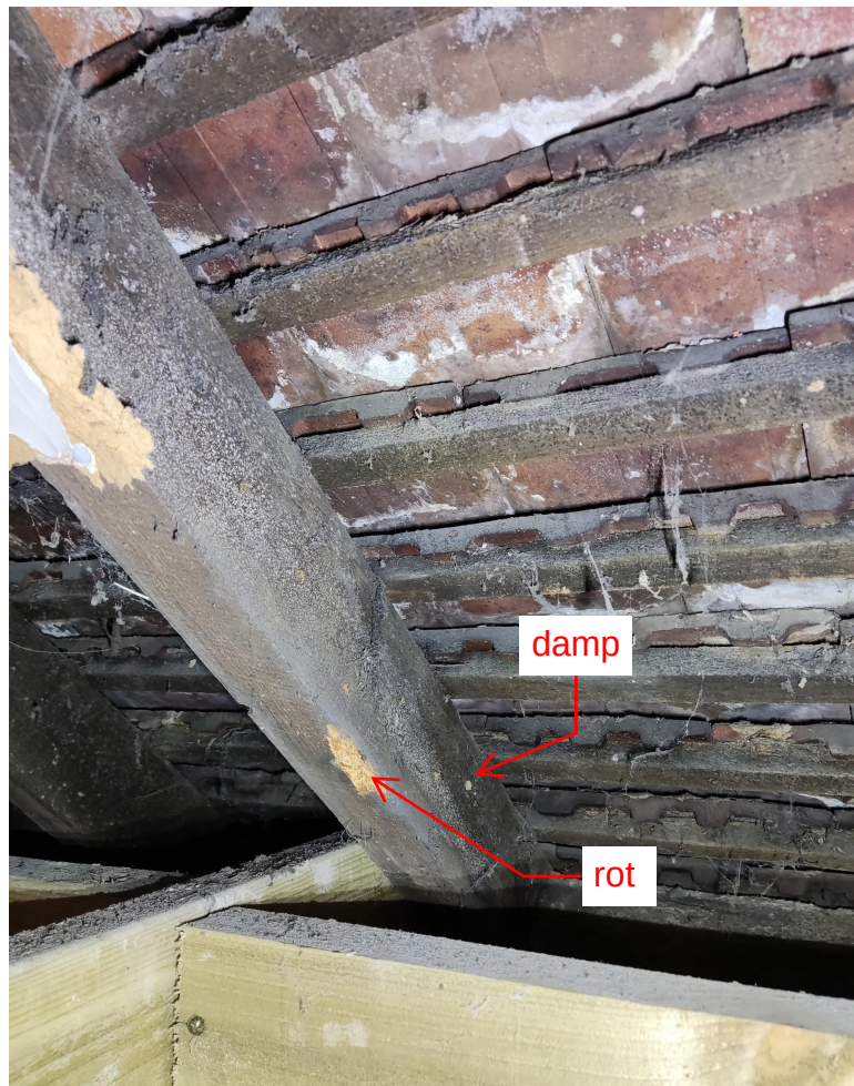
Rafter at frame No.24 is decayed and needs full replacement.
