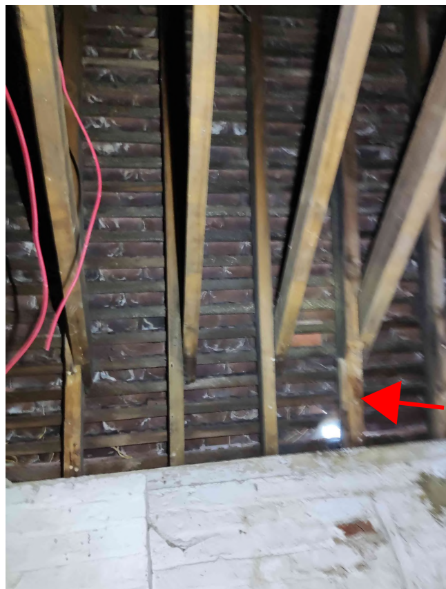
Rafter at frame No.65 is decayed and needs replacement.
