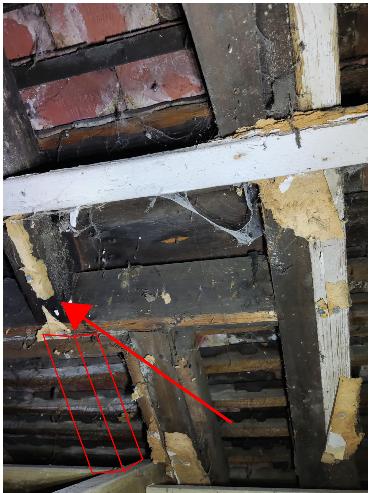
Rafter cut short. It has to be extended to the wall plate at frame No.13.
