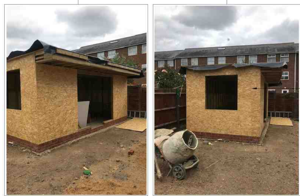
Existing outbuilding; GEFA: 16m 2 Works suspended due to Enforcement notice ENF/346/20
