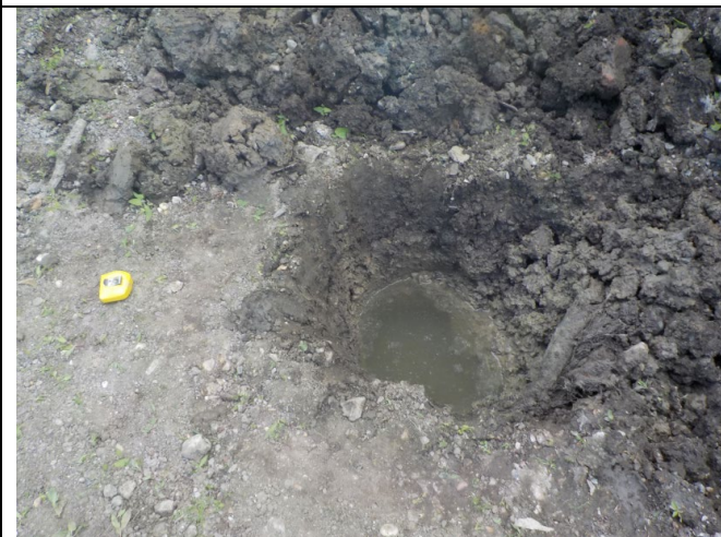
Photo 3 High groundwater encountered in hand dug pits within 'Railway Triangle' area
