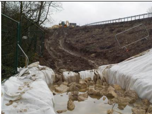
Photo 3 East YB north scour protection and undercut slope toe
