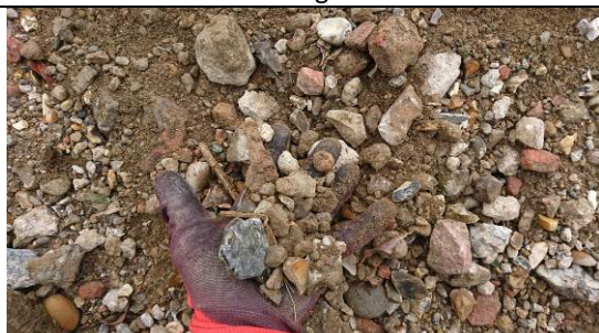
Surface of embankment becoming exclusively gravel as fines are stripped away
