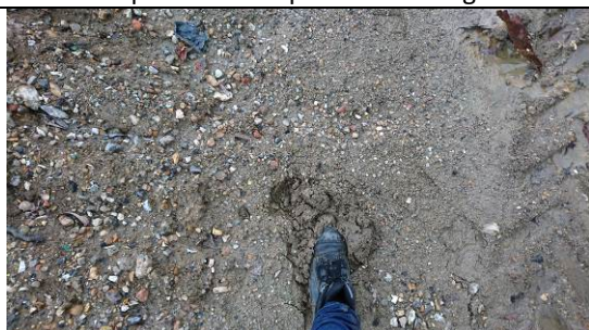
Fines washout accumulating at the embankment toe
