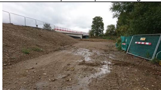
Water emerging/ standing at south embankment toe
