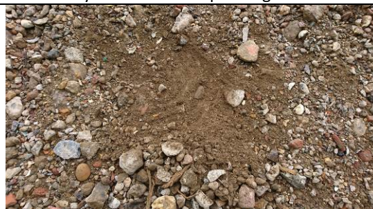
Original embankment finer material visible at depth
