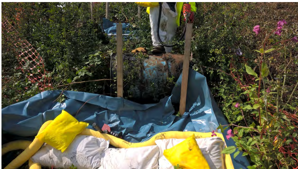
Photo 2. Positioning of spill prevention materials prior to decanting of liquid contents of drums.
