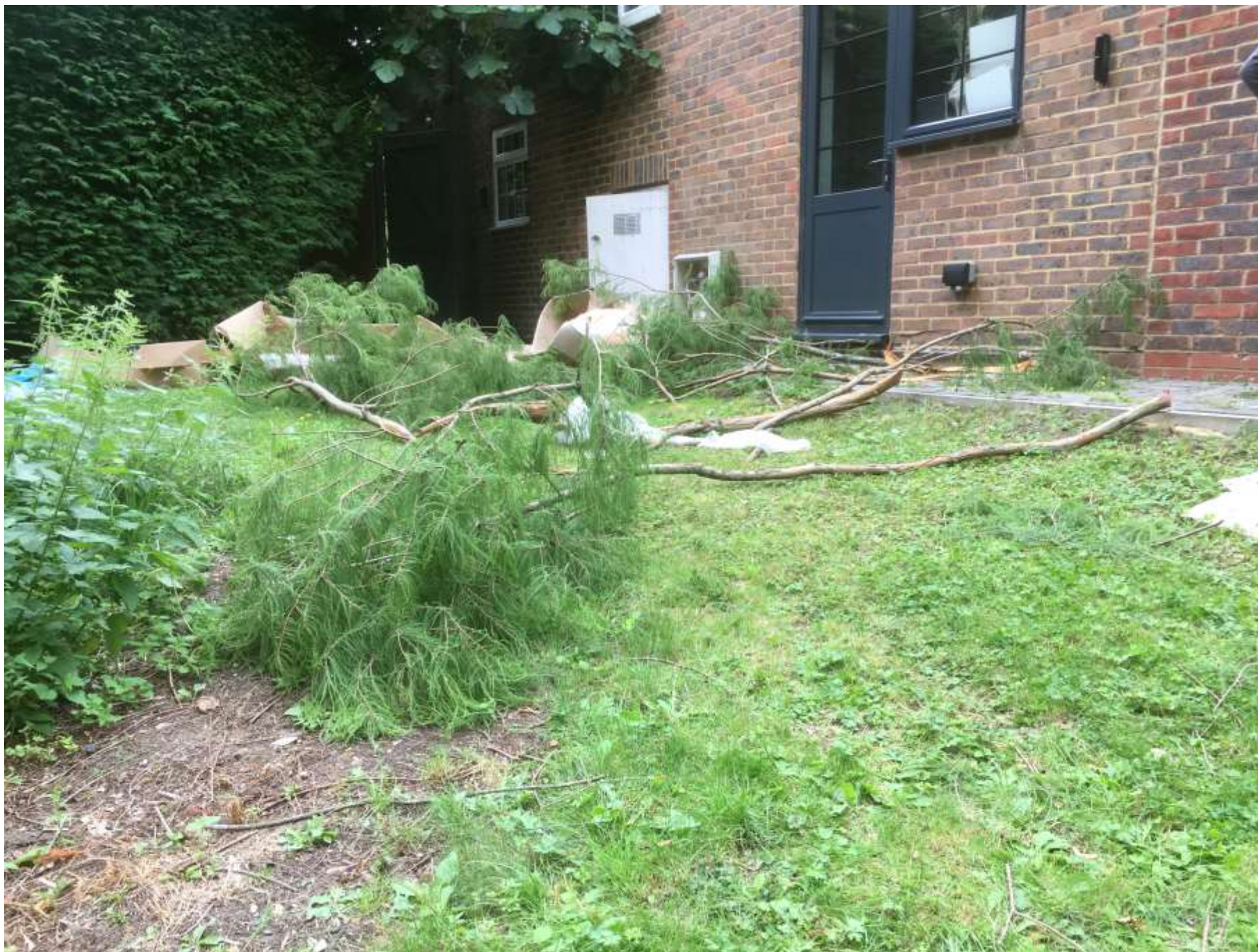
Photo no. 2 to show the 4 x recently failed braches NB Door included for scale and note small branch diameters
