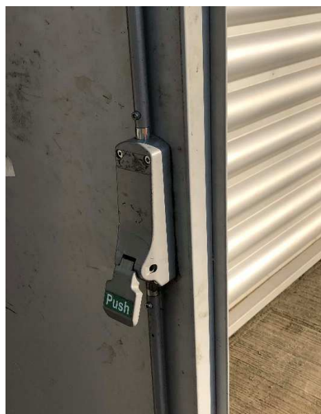
metal security fire door
