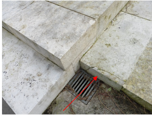
Picture 12. Damage to stone
