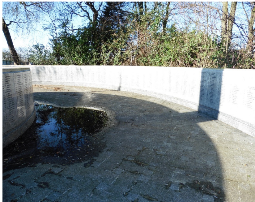
Picture 2. Granite section showing ponding
