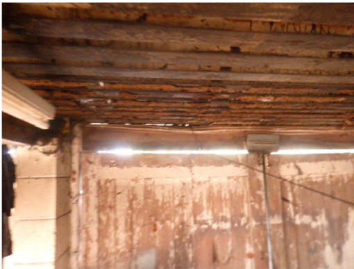
Photograph 25. Unlined roof and daylight over garage doors (internal B2).
