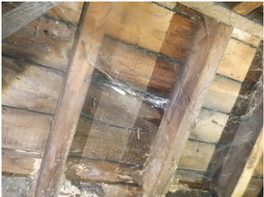
Photograph 23. Tight/intact timber sarking boards that are heavily cobwebbed (B1 - Roof void).
