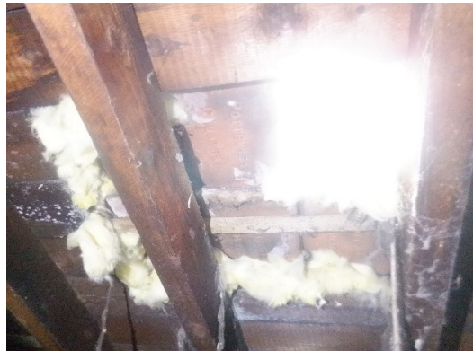
Photograph 24. Blocked skylight with small section of daylight (B1 - Roof void).
