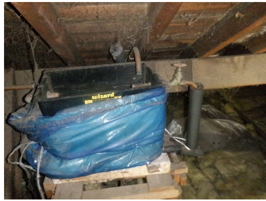
Photograph 22. Small water tank (B1 - Roof void)
