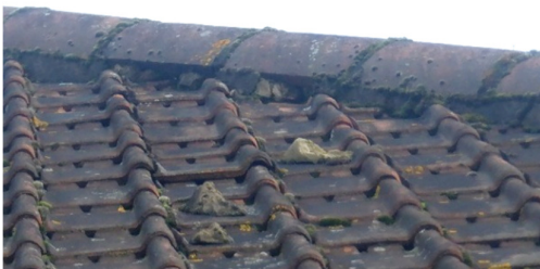
Photograph 17. Superficial gap below crumbling hip mortar (B1 - western elevation).
