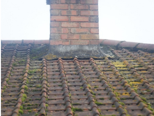
Photograph 18. Lifted lead flashing around chimney (B1 - western elevation).
