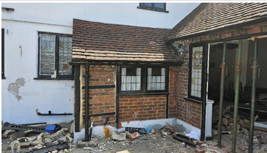
Plate 2. Showing damage on the left-hand side elevation.
