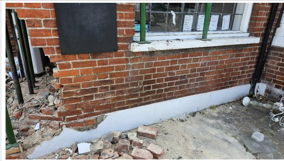
Plate 13. Image showing close up of the damage seen on the right-hand side elevation.
