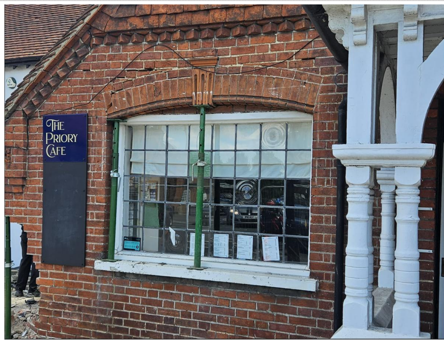
Plate 7. Image showing the damage seen on the right-hand side elevation.
