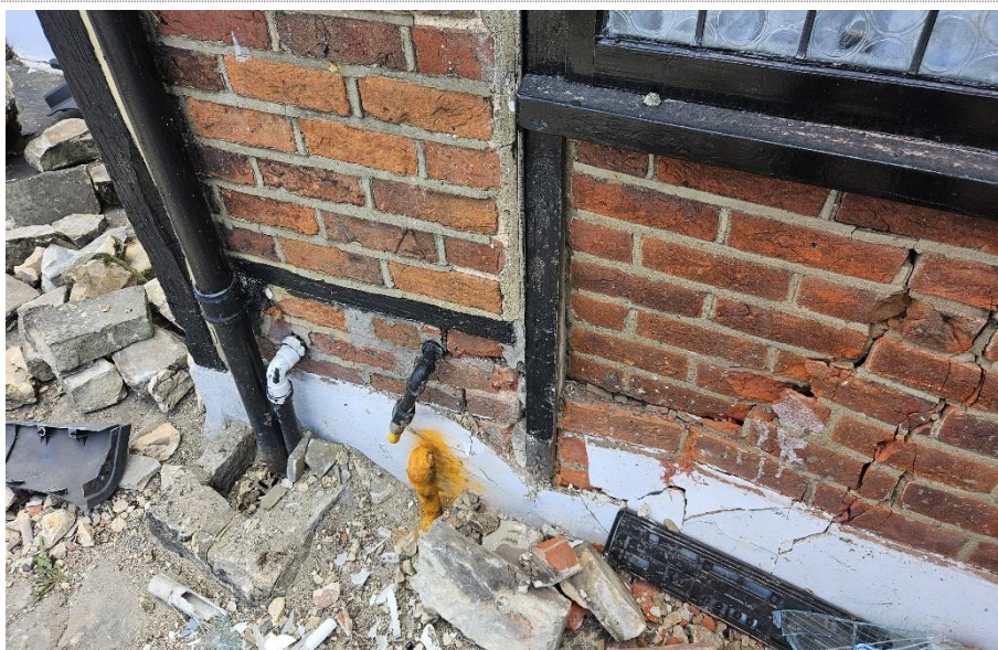
Plate 10. Showing close up of damage seen on the left-hand side elevation.
