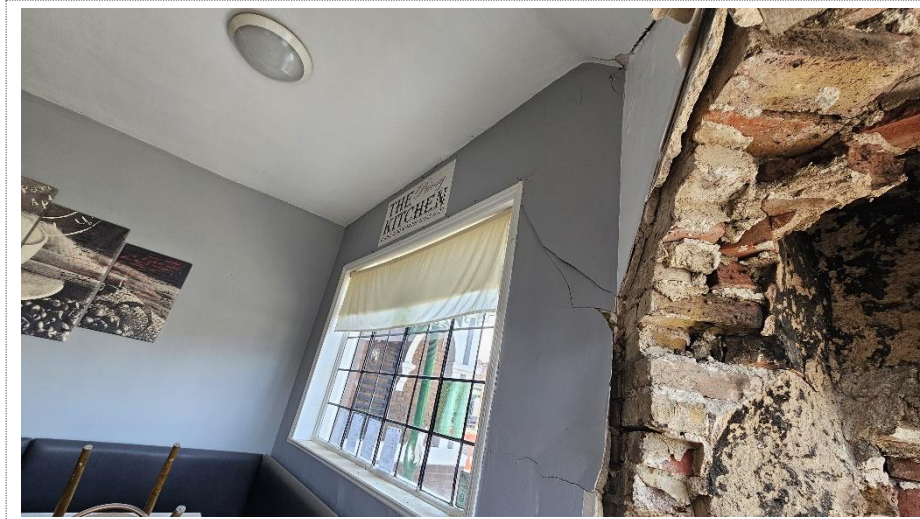
Plate 3. Image showing cracks in the right-hand side elevation.
