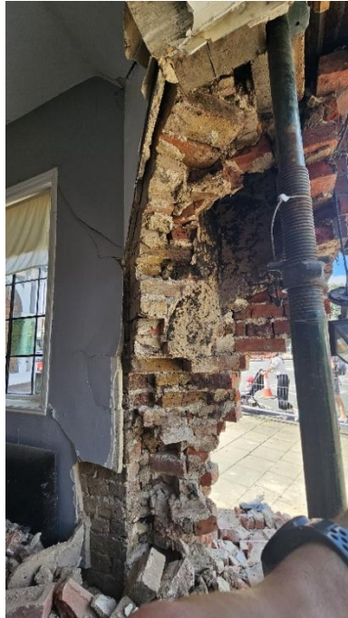
Plate 1. Showing internal damage to the chimney flue and right-hand side elevation wall.
