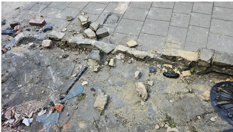
Plate 6. Image showing damaged boundary wall at front elevation.
