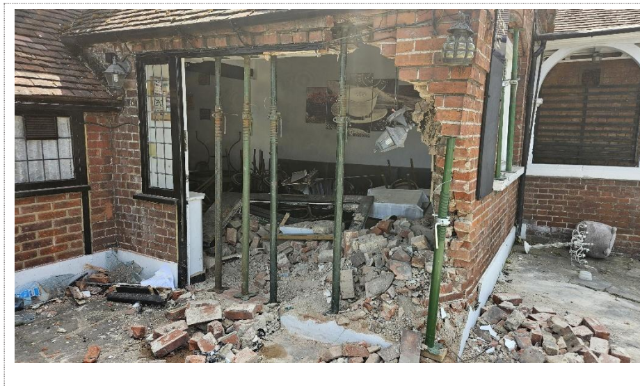
Plate 4. Image showing damaged front elevation.
