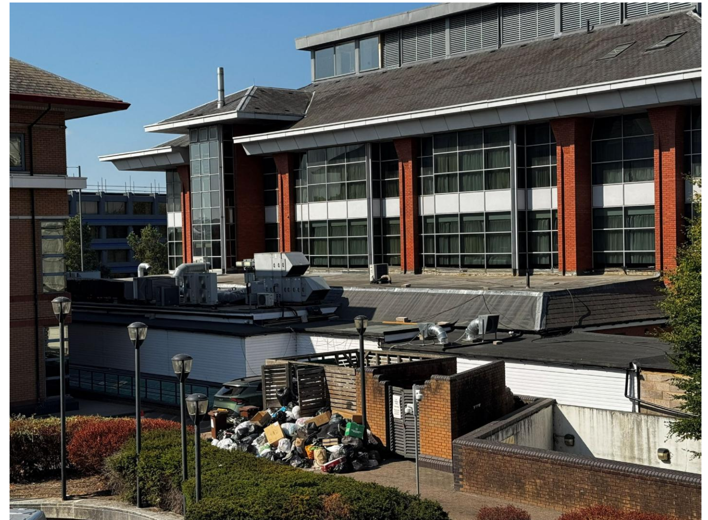
FIGURE 3: VIEW FROM UNATTENDED MONITORING POSITION – LOOKING SOUTHWEST TOWARDS FIXED PLANT SERVING NOVOTEL
